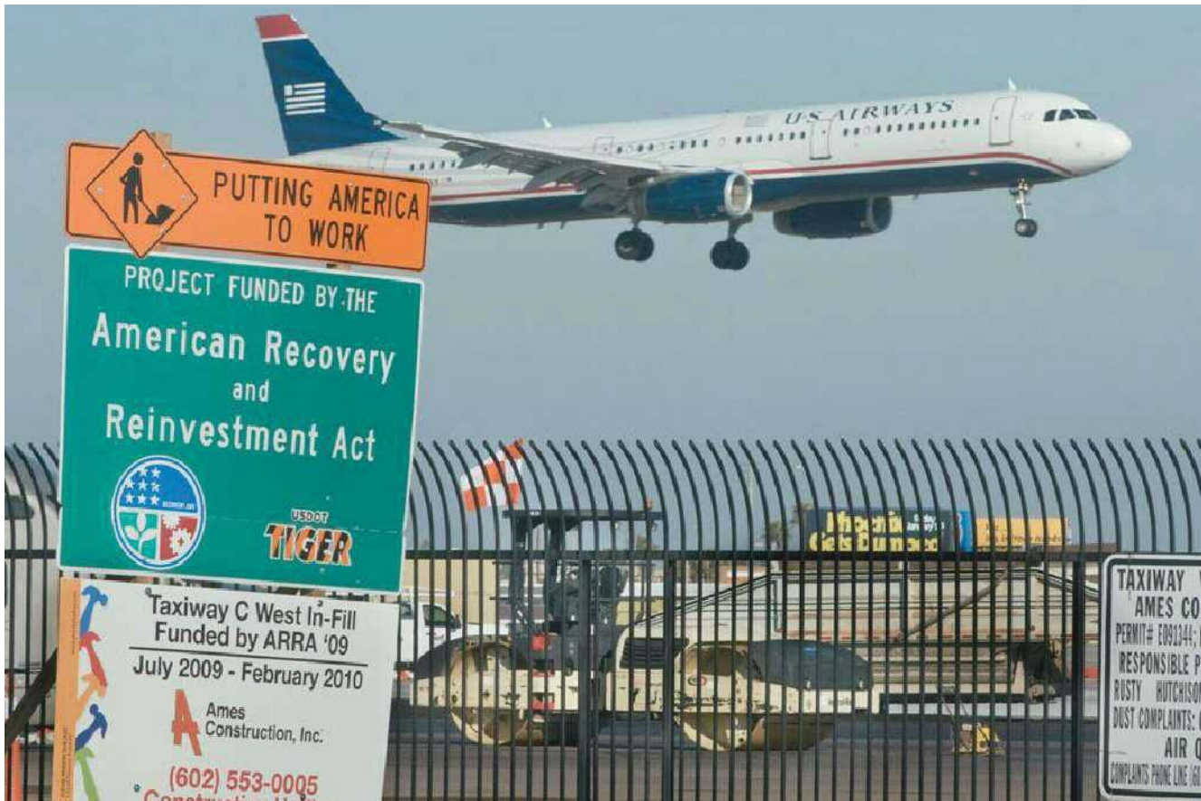
Federal “stimulus” spending Airport construction funded by the American Recovery and Reinvestment Act of 2009. This legislation, known in Washington as the “stimulus package,” was designed to pump $787 billion into the American economy to offset the “Great Recession.” This bill was a decidedly “non-incremental” addition to federal spending and deficits. Indeed, the 2009 federal budget included the largest single increase in spending and deficit levels incurred in any year in history. (© Rick D’Elia/Corbis)
