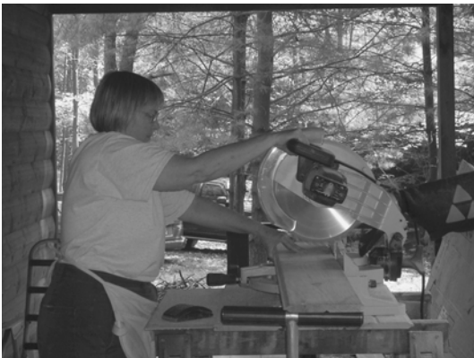
FIGURE 3.1 A woman is using a compound miter saw to cut wood for the interior of a house.
