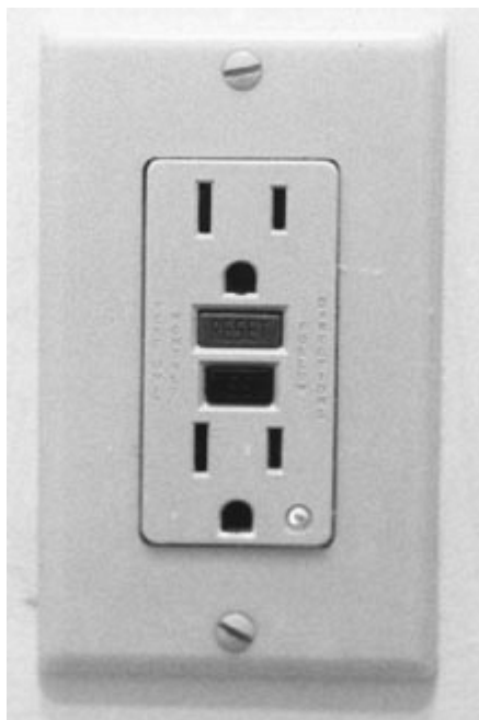
FIGURE 8-28. A GFCI electrical outlet with integrated test and reset buttons.
