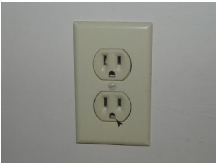
Figure 5-11 Modern electrical outlet in which the ground wire is present. The arrowhead points to the part of the receptacle where the ground wire connects.
