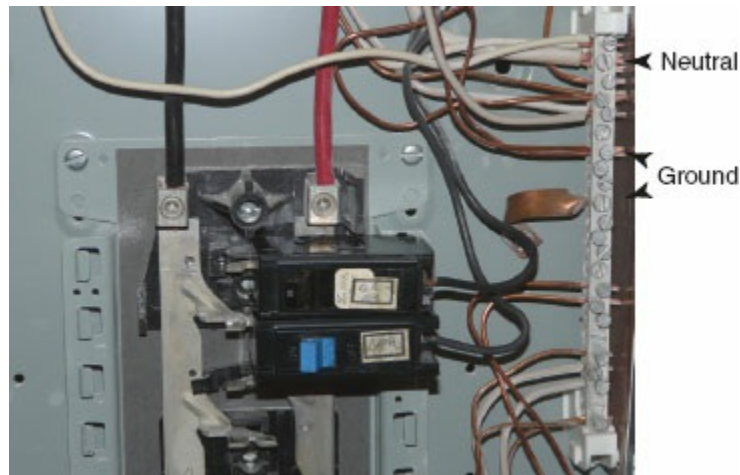
Figure 5-13 The ground wires (bare wires) from the power outlet are run to the neutral bus bar, where they are connected with the neutral wires (white wires) ( arrowheads ).
