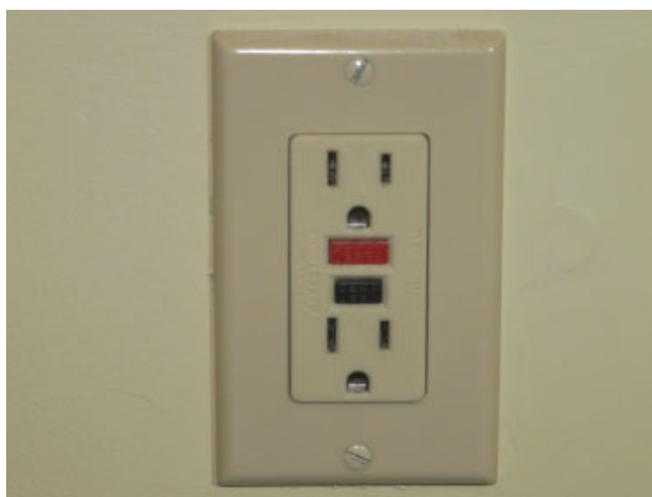
Figure 5-28 A GFCI electrical outlet with integrated test ( black ) and reset ( red ) buttons.
