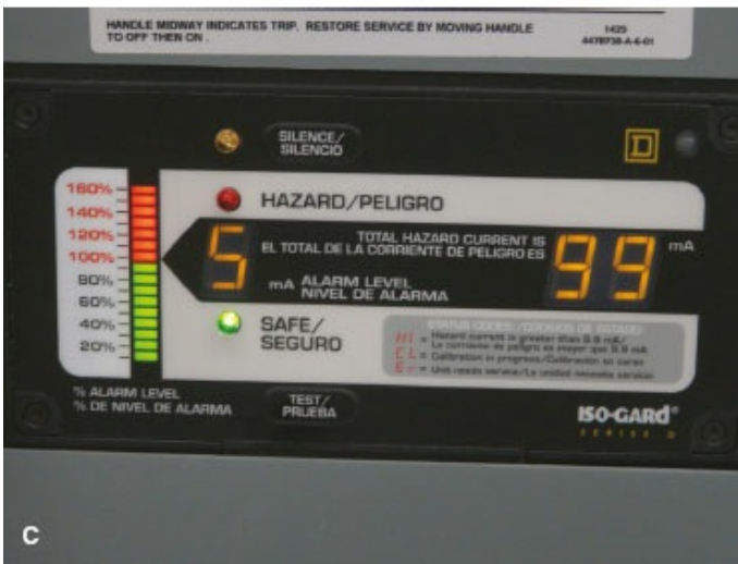
Figure 5-26 The meter of the LIM is calibrated in milliamperes. If the isolation of the power system is degraded such that more than 2 mA (5 mA in newer systems) of current could flow, the hazard light will illuminate and a warning buzzer will sound. Note the button for testing the hazard warning system. A: Older LIM that will trigger an alarm at 2 mA. B: Newer LIM that will trigger an alarm at 5 mA. C: The LIM alarm is triggered, and the red hazard stripe is illuminated, and the number on the right shows 9.9 mA of potential current flow.
