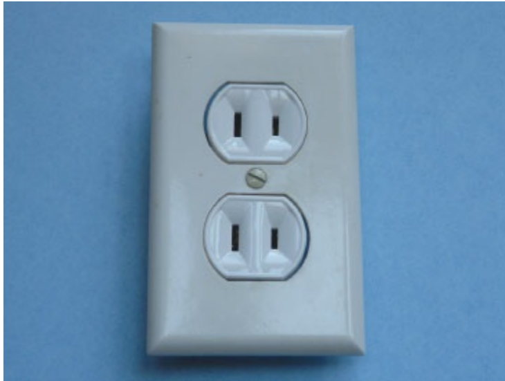
Figure 5-9 An older style electrical outlet consisting of just two wires (a hot and a neutral). There is no ground wire.
