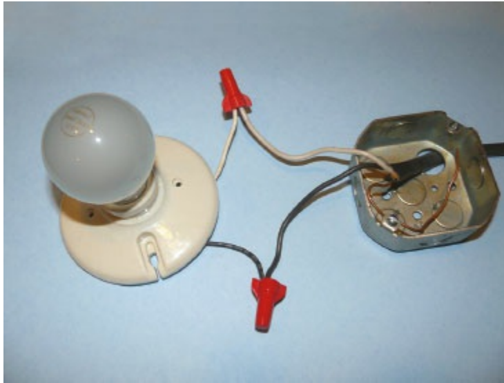
Figure 5-16 A simple light bulb circuit in which the hot ( black ) and neutral ( white ) wires are connected with the corresponding wires from the light bulb fixture.
