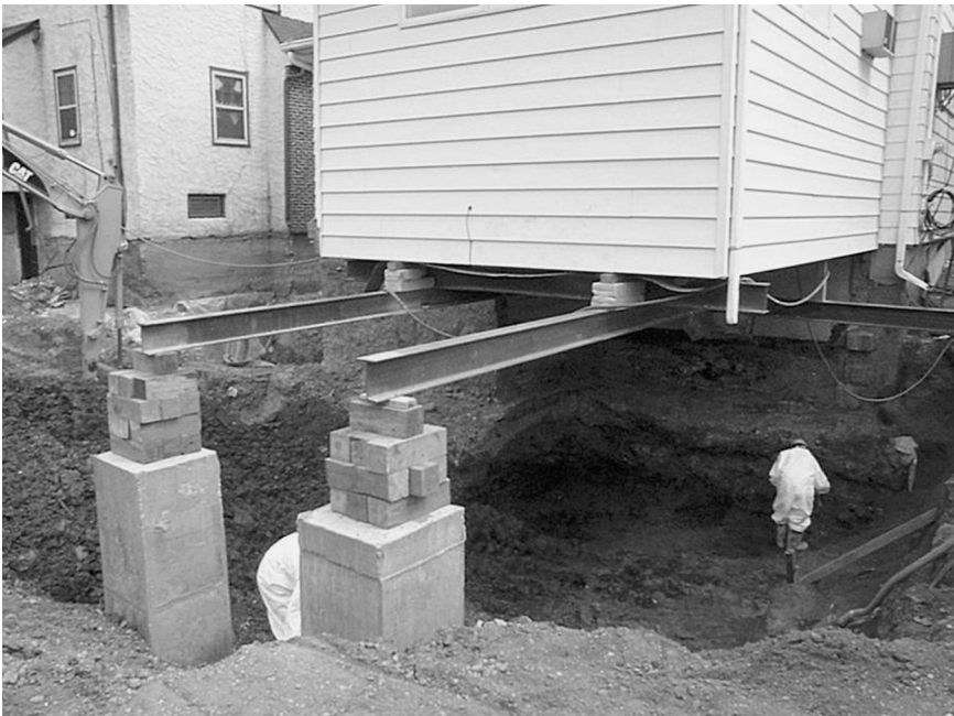
11.1 Lorraine Street home with temporary structural supports during excavation. Technician testing soil post excavation to make sure cleanup goals are met.
