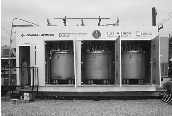
9.4 A transportable fault current controller at the substation in Los Alamos. The picture was taken during testing that occurred after repair of the damage caused by electrical arcing during the initial tests at SCE. (Source: Los Alamos National Laboratory.)
