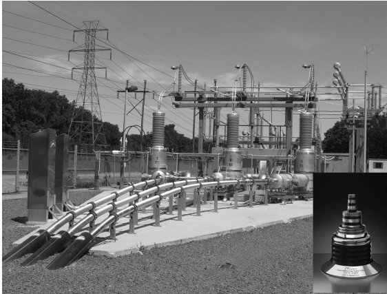
9.22 Terminations for the three phases of the LIPA cable produced by Nexans and AMSC. The installation is on Long Island in New York. The inset shows a cross-section of the cold dielectric cable.
