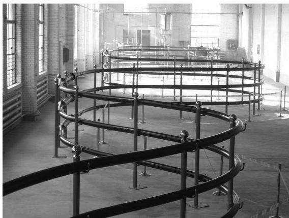
9.24 Test installation of the three phases of the Changtong warm dielectric HTS cable at the Changtong Cable plant in Baiyin, China. This cable is now installed at the 12.5 kV substation in Baiyin city, Gansu province. (Source: Courtesy Changtong Cable.)
