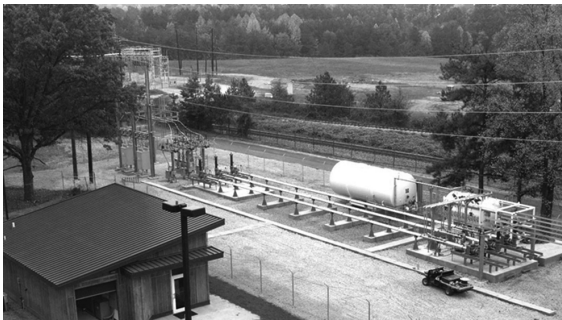
9.23 The first long term superconducting cable installation at the Southwire facility. Southwire is a producer of copper conductors for transformers, cables, etc. This three-phase cable installation delivered power to the plant for over 26000 h.
