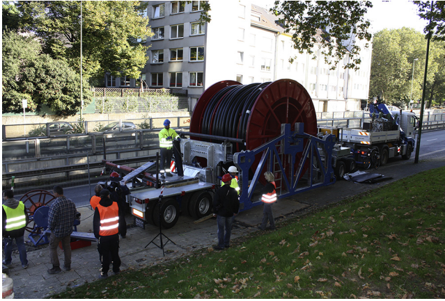
Figure 5.17 AmpaCity HTS AC cable prepared for cable pulling installation in Essen, Germany.
