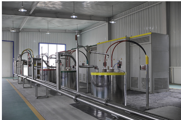
Figure 13.3 A view of the three-phase, 10 kV/1.5 kA high-temperature superconducting fault current limiter.
