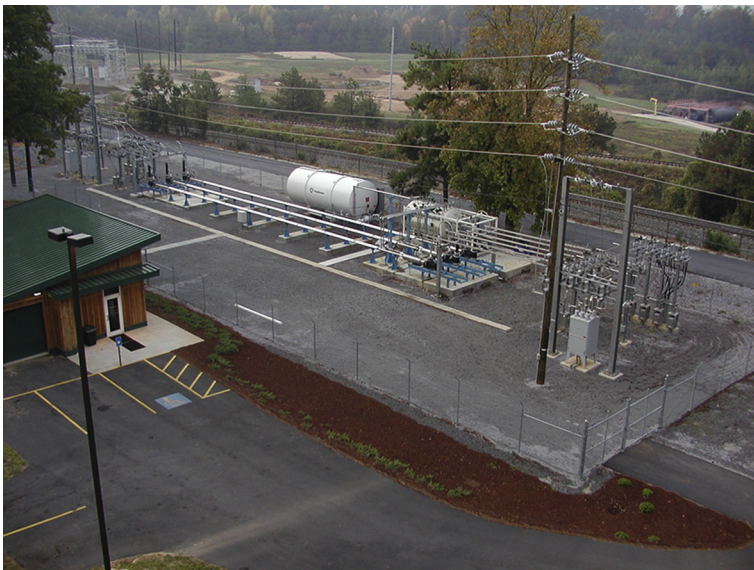
Figure 8.9 The Southwire Co. 30-m HTS power transmission cable and refrigeration system. Photo courtesy of Southwire Co. Carrollton, GA.
