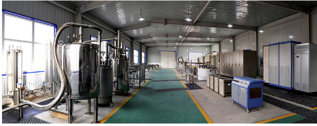
Figure 13.6 A view of the superconducting power substation.
