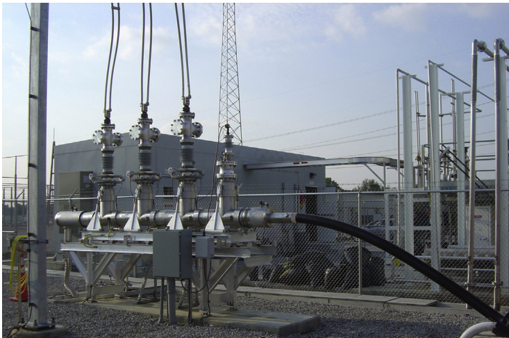
Figure 8.1 Southwire Co. triaxial high-temperature superconducting cable termination installed at the American electric power Bixby substation in Columbus, OH. Photo courtesy of Southwire Co.
