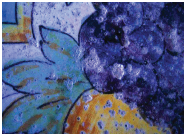
Fig. 1.1 Cracks and pores formed on the surface of a glazed tile (Manises, 18th century) from the floor of the balconies of the Basílica de la Virgen de los Desamparados de Valencia, Spain
