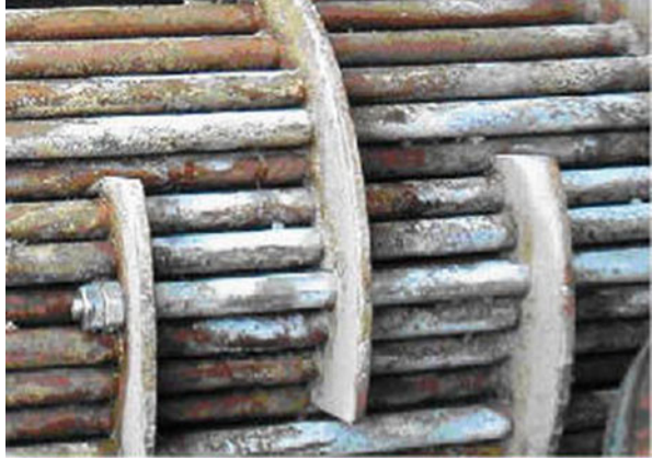
Fig. 3.2 Scaling on heat exchanger surfaces. (Reproduced with permission of H&C Heat Transfer Solutions)
