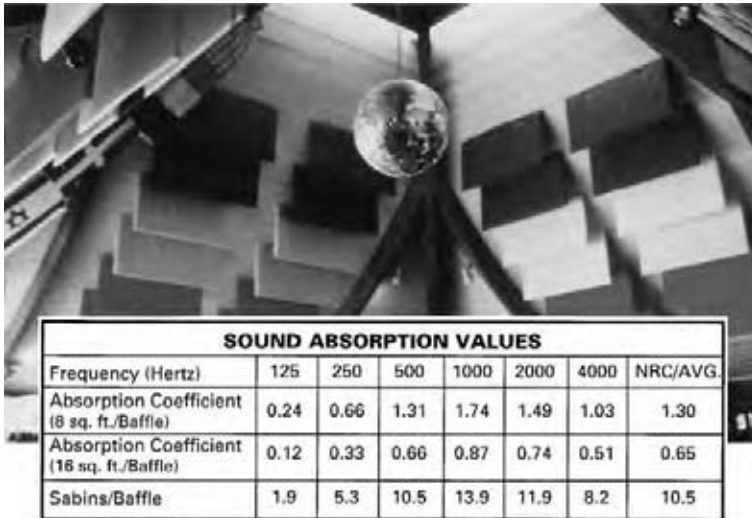
Fig. 19.7 Application of hanging acoustic baffles to reduce reverberation in the high pyramid-shaped ceiling of a restaurant. The baffles are 1½-in.-thick (38-mm) fiberglass with a tough fire-rated cover. Sound absorption values are given in the accompanying table. (Courtesy of The Proudfoot Co., Inc.)
