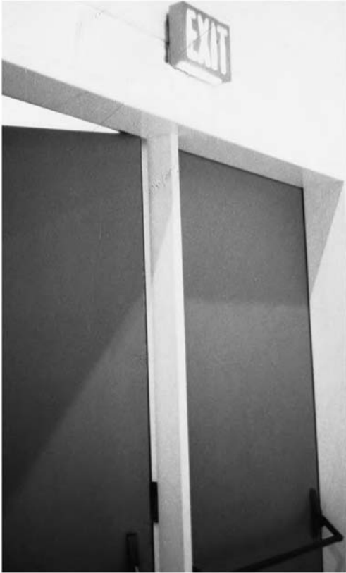
Fig. 16.33 Typical application of an exit light with a built-in battery, charger, and controls. Note that the bottom of the unit is designed to illuminate the area immediately in front of the exit. (Photo by B. Stein.)
