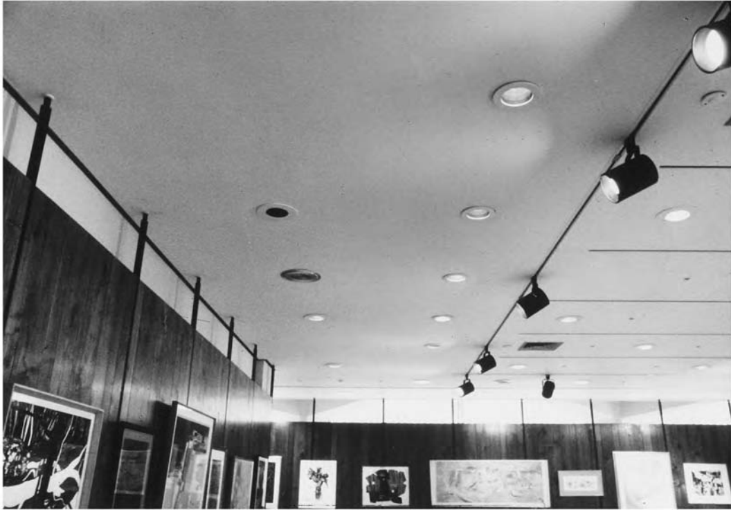
Fig. 16.9 Art exhibition room illustrating good and bad lighting techniques. The upper wall fenestration is excellent for deep daylight penetration. Track lighting is ideal for display of art. The mixture of incandescent downlights for general lighting is excessive and an eyesore. Also, the positioning of the track lights can create both direct and reflected glare problems and annoying shadows unless the sources are selected properly and ceiling height is at least 10 ft (3.1 m).
