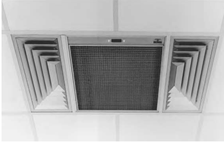
Fig. 5.25 A stand-alone electrostatic air filter operates independently of the central HVAC system; no ductwork is required. Airflow rates vary; the slower the flow, the more efficient the filtering. Flush-mount (recessed in suspended ceiling), ceiling surface-mount, wall-mount, and portable models are available. (Courtesy of Tectronic Products Co. Inc., East Syracuse, NY.)
