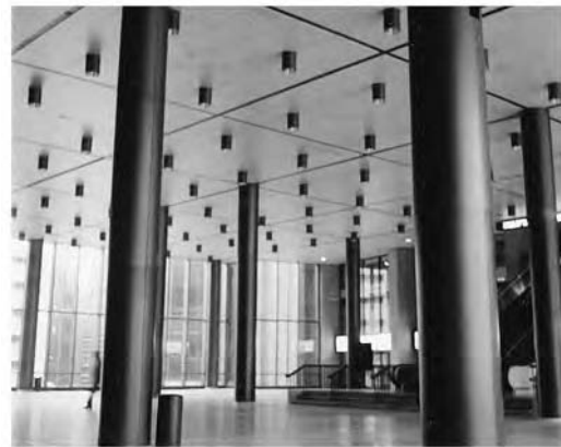
Fig. 13.17 The large, can-shaped, surface-mounted downlights dominate the area's appearance despite the high ceiling.
