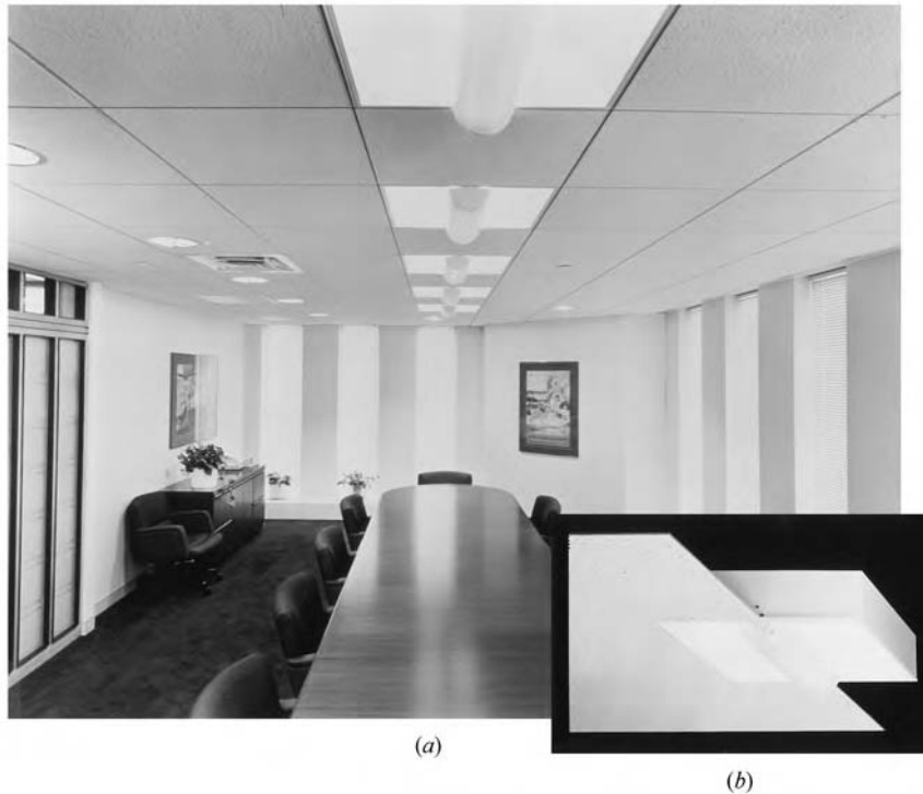
Fig. 16.23 Luminaire construction giving a direct-indirect appearance (a) using a direct troffer construction (b). The medium-brightness luminaire interior reflects light, giving a deep, airy appearance. The translucent lamp enclosure maintains an acceptable luminance against the background (interior) reflector. The photometric characteristic is essentially circular in both longitudinal and transverse planes. (Courtesy of Zumtobel-STAFF Lighting Co.)
