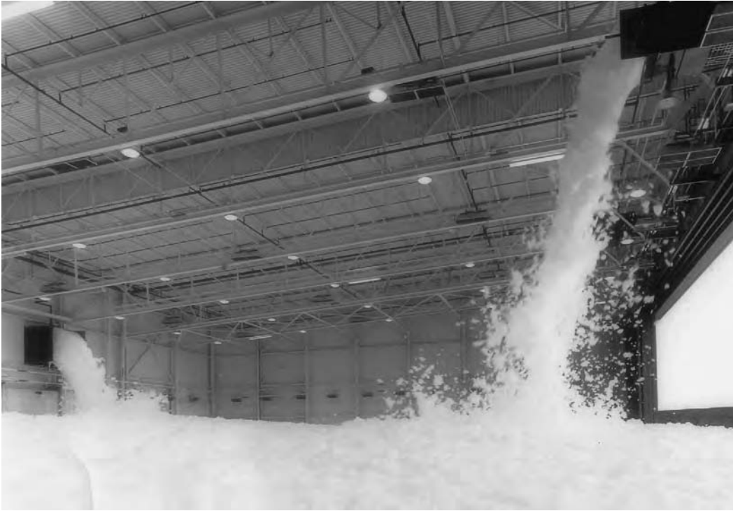
Fig. 24.27 Detergent foam (high-density) discharged from four units (two of which are seen in the illustration) after 3 minutes of operation. This installation at a hangar building at Detroit Metropolitan Airport smothers fire, prevents its spread, and will not harm airplanes or machinery. The system can handle combustible liquid fires. (Note also the supplementary grid of upright sprinklers directly below the roof surface.)
