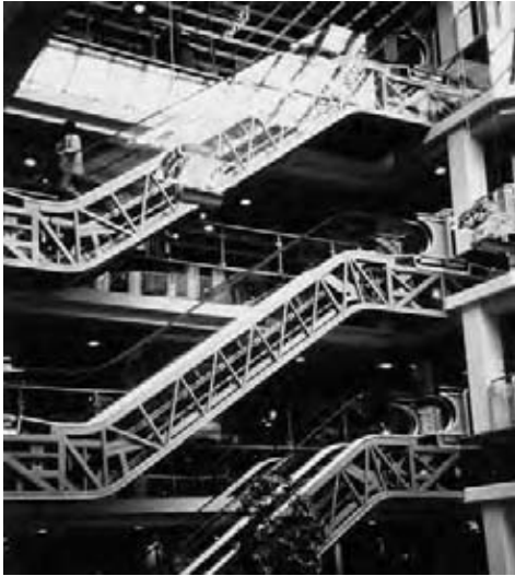
Fig. 33.6 An unusual design of stacked parallel escalators with a forced walk-around in a continuous trip. The exposed truss and drive elements, combined with a transparent balustrade, add considerable visual interest to the installation. (Photo courtesy of O&K Rolltreppen, Germany.)
