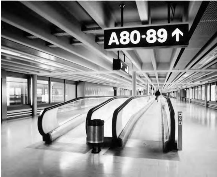
Fig. 33.19 Twin autowalks in a transportation terminal. Of particular interest are the sloped entry and exit and the continuous fluorescent lighting beneath the handrails of the balustrades. (Photo courtesy of O&K Rolltreppen, Germany.)
