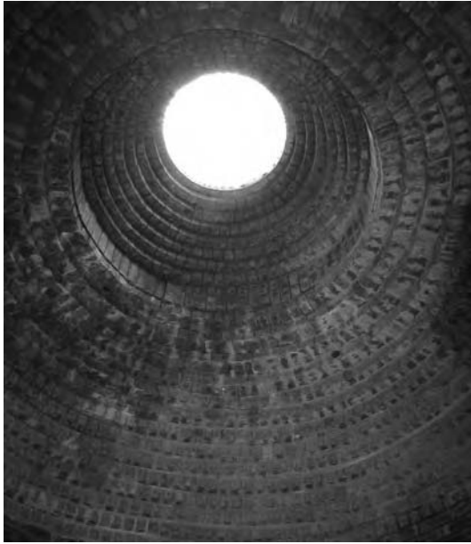
Fig. 20.28 Oculus of the water tower cistern. The tower serves as a focal point for views of the site. (Photo by Jake Moore; © 2009 Alison Kwok; all rights reserved.)
