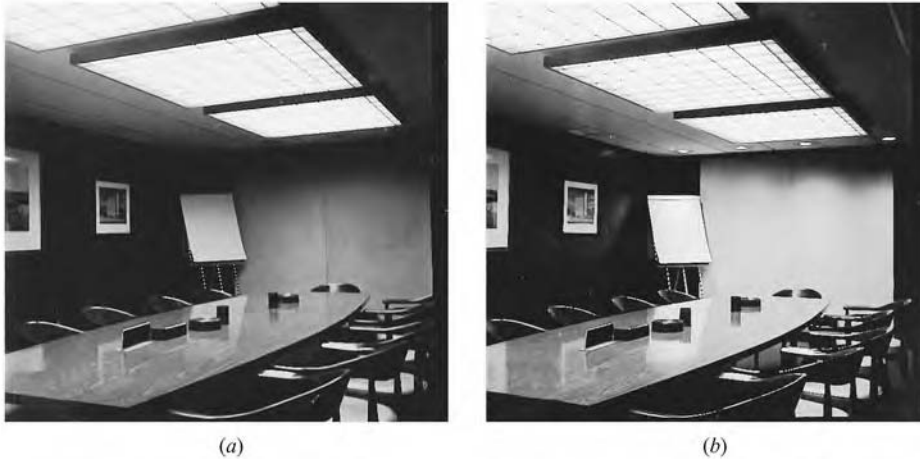
Fig. 13.11 Large-dimension lighting fixtures may be used in a low-ceilinged room if the apparent size of the unit is reduced. Here at a mounting height of 7 ft 6 in. (2.3 m), 4 \times 4 -ft ( 1.2 \times 1.2 -m) units are acceptable because the lattice on the face of each unit gives the impression of reduced fixture size. Note also that the apparent illumination in (b) is greater than in (a)—although both are exactly equal on the table surface—due to the wall wash in the background. The eye perceives vertical surface illumination more readily than horizontal illumination and retains the impression for the entire space.
