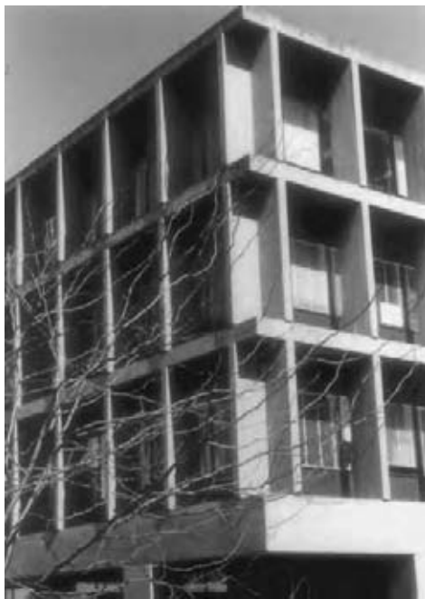
Fig. 3.19 The "eggcrate" shading devices shown on the southwest corner of this University of Oregon building reduce solar heat gains by blocking acute sun angles from either side of the window. Different shading devices are appropriate for different façade orientations.
