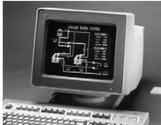
Fig. 30.32 Workstation screen shows a portion of a building system and the status of all components. Here we see the chiller status (on-off, COP, tons, run time), water temperature and flow in supply and return lines, and condenser water temperature. (Courtesy of Johnson Controls.)
