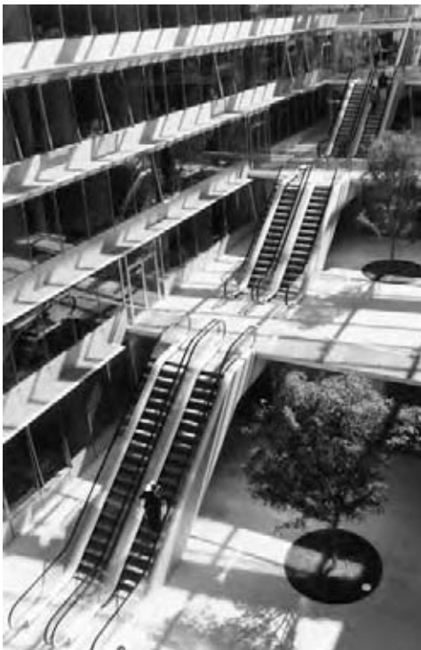
Fig. 33.7 An unusual installation of parallel escalators adapted to a long four-story building. In the more common instance of a building that is taller than it is long, the escalators are stacked as in Fig. 33.6. Here the design is adapted to the large central court/atrium, with offset stepped landings and entrances to the buildings. (Photo courtesy of O&K Rolltreppen, Germany.)
