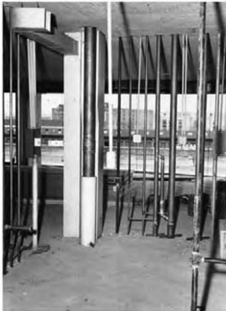
Fig. 22.26 Plumbing risers in a fireproof multistory building. Pipes, tubes, conduits, and ducts adjoin toilet rooms and utility spaces. Ventilation ducts and a master 5-in. (127-mm) copper hot-water riser are just to the left of center. Soil and vent stacks with hot and cold water supplies, all of copper, are to the right of this group. At the left, in a lighter tone, are the galvanized steel feeder conduit and distribution circuit conduits for a local electrical control panel box. Note that some pipes and tubes are supported at this floor by bolted clamps. After testing and before pipes are enclosed, covering will be completed. (Courtesy of Copper Development Association.)
