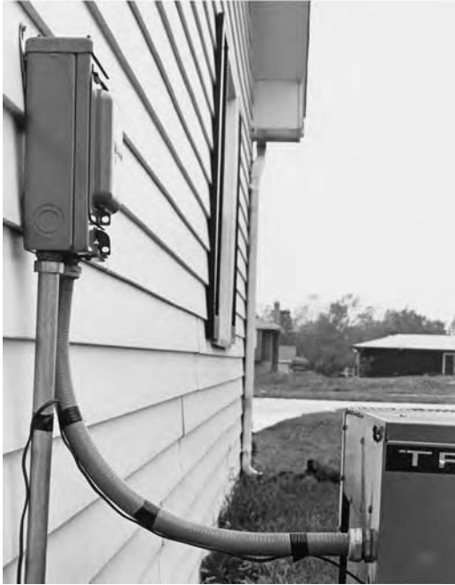
Fig. 27.18 This is a particularly good application of liquid-tight, flexible conduit because it provides weatherproofing and mechanical isolation of the vibration-producing equipment. (Courtesy of Electri-Flex Company.)
