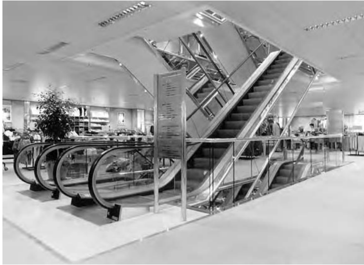
Fig. 33.4 Crisscross design applicable to either spiral or walk-around operation. The horizontal area in the right foreground can be used to display impulse-buying merchandise to walk-around riders during holiday seasons, after which operation can be returned to the spiral mode. (Photo courtesy of O&K Rolltreppen, Germany.)
