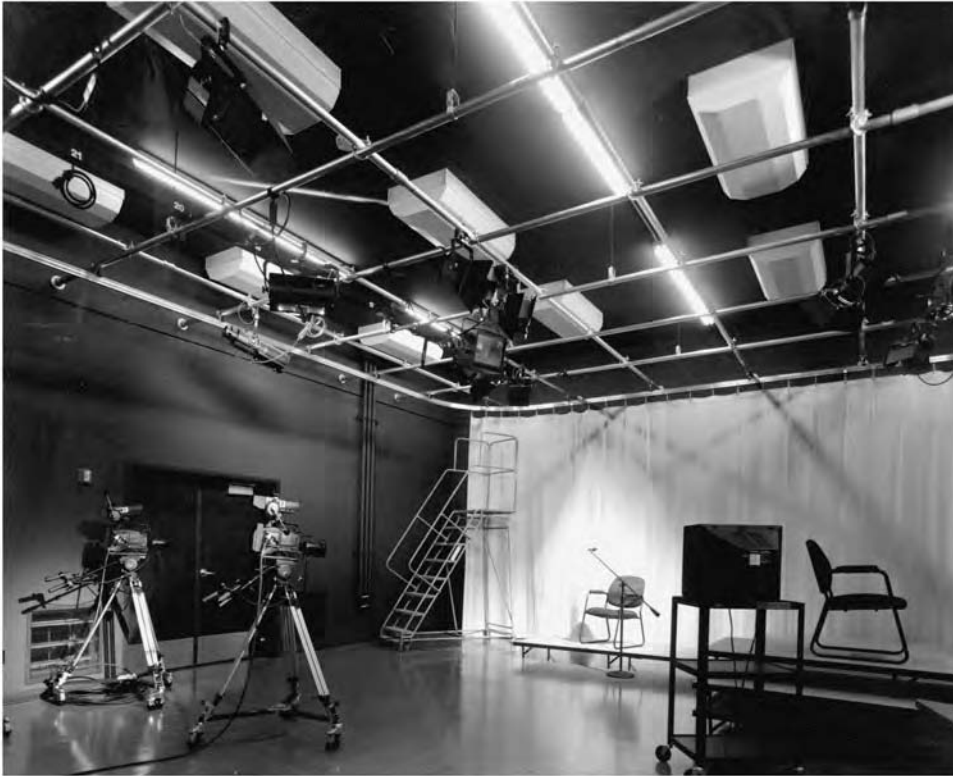
Fig. 10.47 Pinhole-perforated diffusers (above a lighting grid) provide large quantities of low-velocity air to the television studio at the Community Media Center of Santa Rosa, California. The background noise from more typical HVAC systems would be amplified by sound recording equipment and hence would be unacceptable. (© TLCD Architecture, Santa Rosa, CA.)
