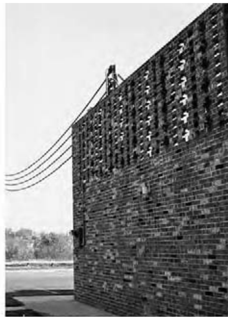
Fig. 26.6 (a) Pad-mounted exterior transformers are neat, compact, and, if sited properly, unobtrusive. Large units can be partially screened by shrubbery. (b) When the size is such that visual screening becomes a problem, consideration should be given to a structural screen such as a decorative brick wall. (Courtesy of General Electric, U.S.A.)
