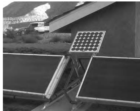
Fig. 29.16 Synergistic PV application—pumping hot water produced by solar collectors for a residence in the Southwestern United States. (Photo ©2004 by Walter Grondzik; all rights reserved.)
