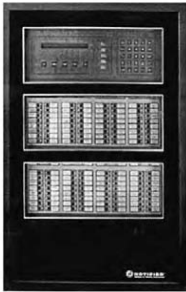
Fig. 24.64 Large addressable analog (intelligent) fire alarm control panel, suitable for network connection, computer interface, and operation in conjunction with an emergency voice/alarm communication system of the type used in multistory office buildings (see Fig. 24.65). The unit can accommodate 990 analog detectors and an equal number of monitor/control modules. It is illustrated with a 96-point integral annunciator, and additional annunciation can be connected. The integral control panel provides for polling, diagnostics, sensitivity control of all detectors, automatic detector drift compensation, alarm verification, front-panel programming, and options for system connections, as shown in the block diagram of Fig. 24.63. (Photo courtesy of Notifier, division of Pittway Corp.)
