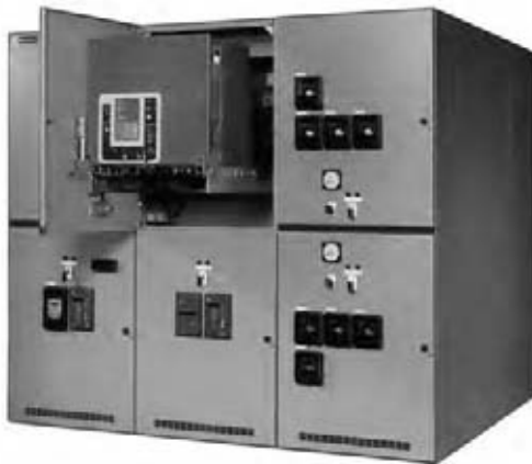
Typical indoor assembly with a breaker withdrawn on rails
