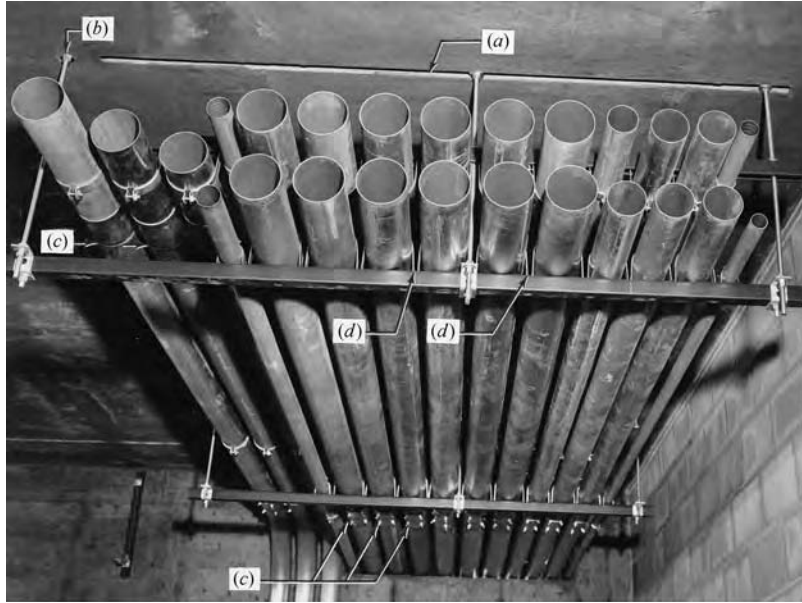
Fig. 27.17 Typical overhead conduit bank installation. Note that due to field conditions the insert (a) for hanger rods was inadequate and an additional insert (b) was added. This conduit bank uses EMT, which has a pipe-wall thickness approximately one-third that of heavy-wall rigid conduit. The resulting weight difference in a large bank such as this is very pronounced. EMT joints are made with set-screw fittings (c). Note how individual conduits are fixed by clamps to the trapeze channel (d). (Courtesy of Republic Steel Corp.)
