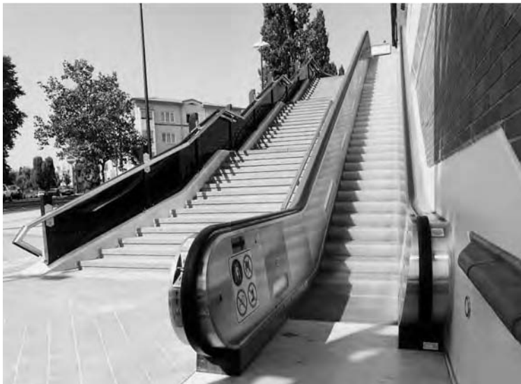
Fig. 33.16 An all-weather exterior electric stairway is often the best solution to an elevated building entrance or exit. Note the elongated left balustrade, which prevents bunching at the escalator entrance, and the fluorescent fixture built into the balustrade, which provides nighttime step lighting. (Photo courtesy of O&K Rolltreppen, Germany.)
