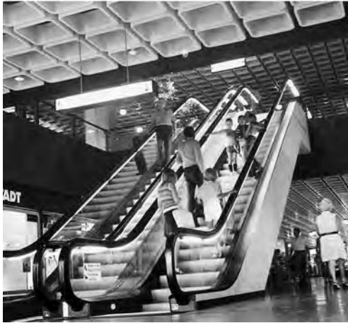
Fig. 33.15 A continuous fluorescent source is placed under the handrail of the crystal balustrade in this covered mall in West Germany. Note the additional light at the base for illuminating the combplate. (Photo courtesy of O&K Rolltreppen, Germany.)
