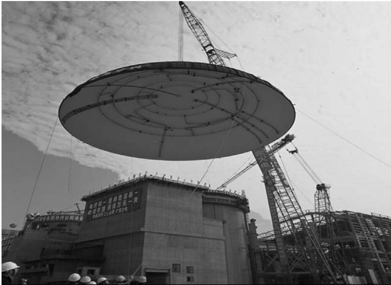
9.2 Modular construction at Lingao (China), the containment dome was assembled on the ground at the site and installed as a single module (weight 143 tons, diameter 37 m, height 11 m).
