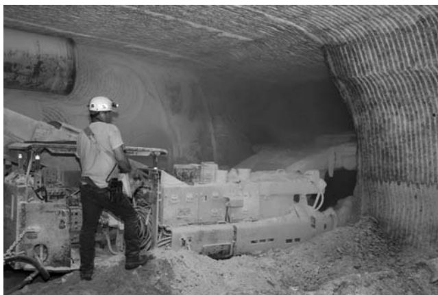
14.10 The Waste Isolation Pilot Plant uses a continuous miner to carve disposal rooms out of the Permian Salt Formation, nearly a half mile below the surface (© US DOE).
