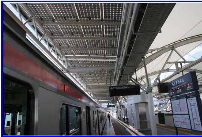
Figure 6. Light-through PV systems in Motosumiyoshi Railway Station, Kawasaki City, Kanagawa Prefecture.
