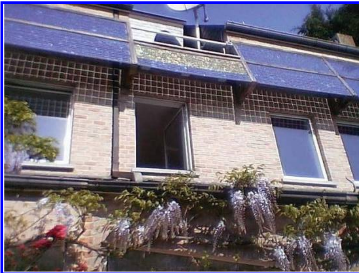
Figure 36. W. Palz's residence in Brussels. The 1-kW PV plant was the first to be installed in Europe's capital in 2000, without a subsidy. The array also has some coloured cells from Japan. The support structure is untreated timber.
