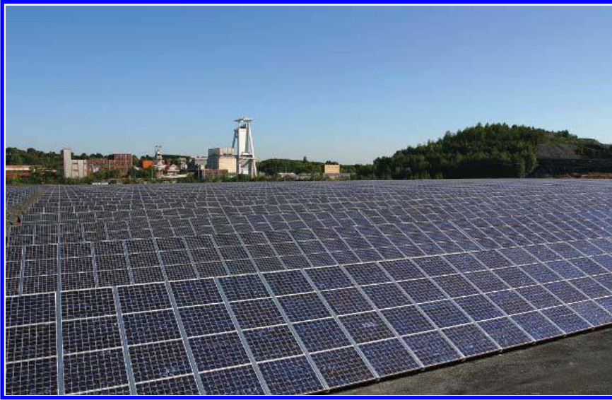
Figure 63. The bright solar future: a large PV plant in front of a coalmine in Saarland (W. Palz's home state), Germany.
