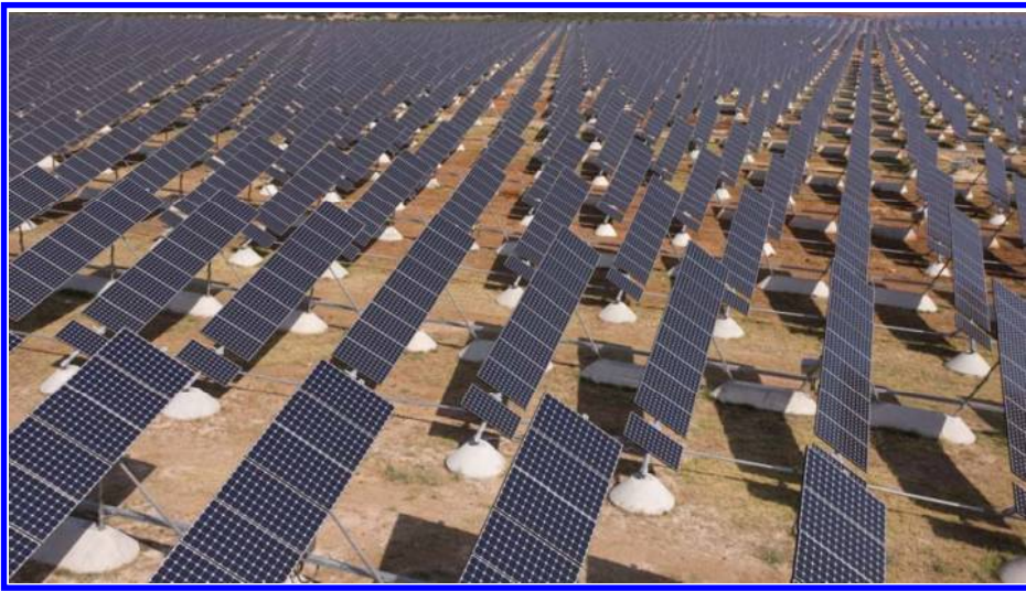
Figure 5. Large SunPower PV power plant using tracking structures to follow the sun.
