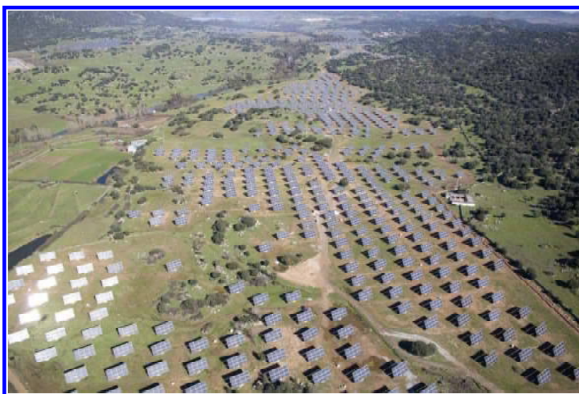
Figure 1. 10 MW 2-axis tracking flat panel PV power plant at Jerez de los Caballeros (Spain).
