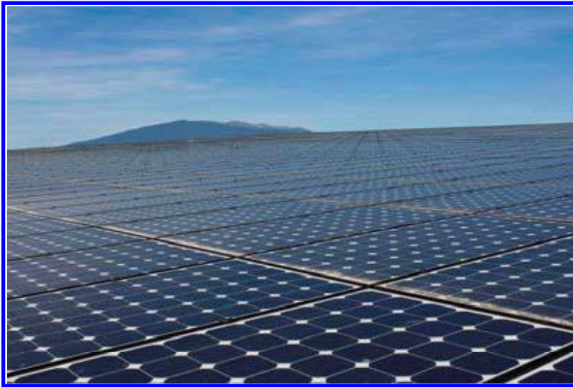
Figure 49. SIG/SES-Société d'énergie solaire SA, 1228 Plan-Les-Ouates, Zurich/Basel, was awarded the Swiss and European Solar Prize in 2008. In 2008/09, the 571 kWp PV installation with Sunpower solarcells produced on the average 585 000 kWh/a. With a surface of 3395 m 2 , this results in 172 kWh/m 2 a, which is enough to drive 15 000 km each with 400 solar-powered electric cars each year (see Swiss Solar Prize 2008, front page and p. 34/35).
