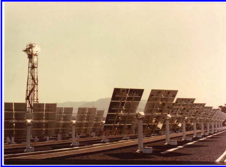
Figure 25. The field of heliostat mirrors and the receiver tower at Eurhelios.
