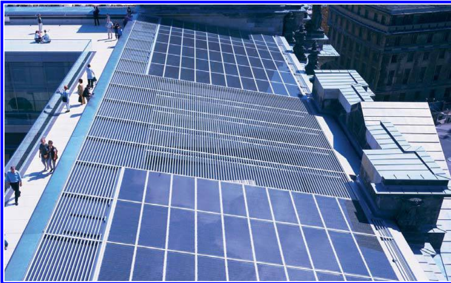
Figure 7. Photovoltaic cells on the south-facing section of the Reichstag's roof power a moveable sunshade in the cupola. The shade is suspended on rails allowing it to track the path of the sun. In addition, the photovoltaic cells drive mechanical fans within the cone to help facilitate airflow.
