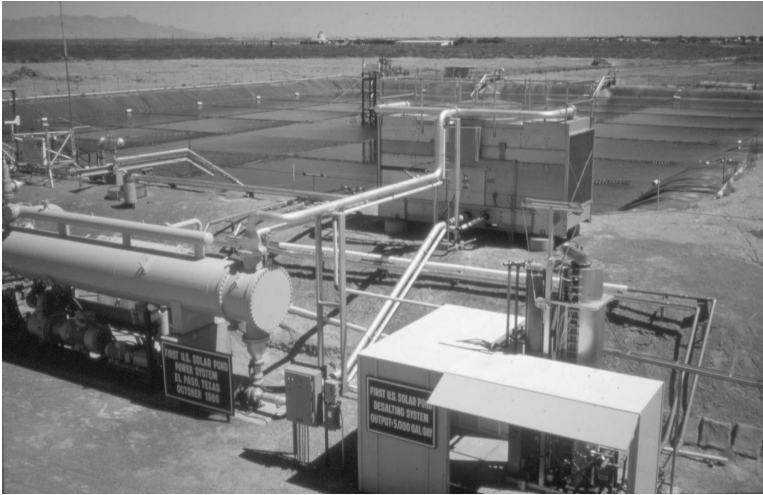
FIGURE 7.20 El Paso solar pond with Rankine-cycle engine (100 kW) for electric generation in the foreground.
