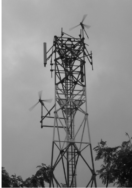
FIGURE 9.19 Two 1.5-kW wind turbines at telecommunication system, China. (Courtesy of Charlie Dou.)
