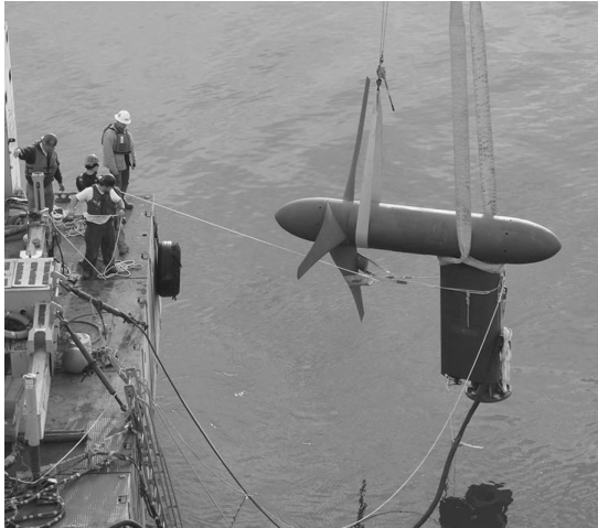
FIGURE 12.15 Tidal turbine, 35 kW, being installed in East River, New York City. (Courtesy of Verdant Power.)
