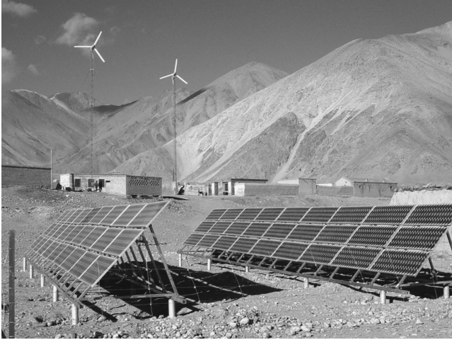
FIGURE 15.3 Hybrid system (54 kW) for village power, Subashi, Xingiang Province, China. (Courtesy of Charlie Dou.)
