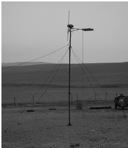
FIGURE 9.16 Small wind turbine, 50 W, isolated household, Inner Mongolia, China. Notice rope on tail for manual control; however, this control mechanism is not recommended by manufacturer.
