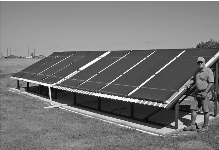
FIGURE 5.20 Solar hot water system for heating a swimming pool. Fixed tilt angle of array is 27^\circ for summer sun at 35^\circ N. Eight panels, thermoplastic, each 1.2 by 3 m (4 by 10 ft).
