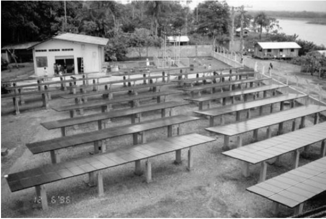
FIGURE 6.17 A 50-kW PV array with controller and a large battery bank were added to the diesel station in the village of Campinas, Amazonas, Brazil. (From National Center for Photovoltaics, National Renewable Energy Laboratory (NREL), www.nrel.gov/ncpv .)
