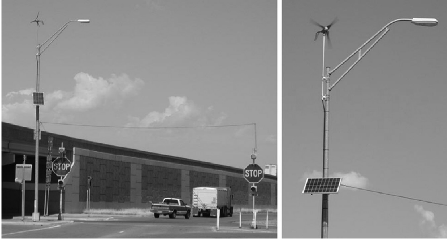
FIGURE 9.20 PV-wind powers streetlight and flashing red lights at stop signs, McCormick Road on I27 between Canyon and Amarillo, Texas.
