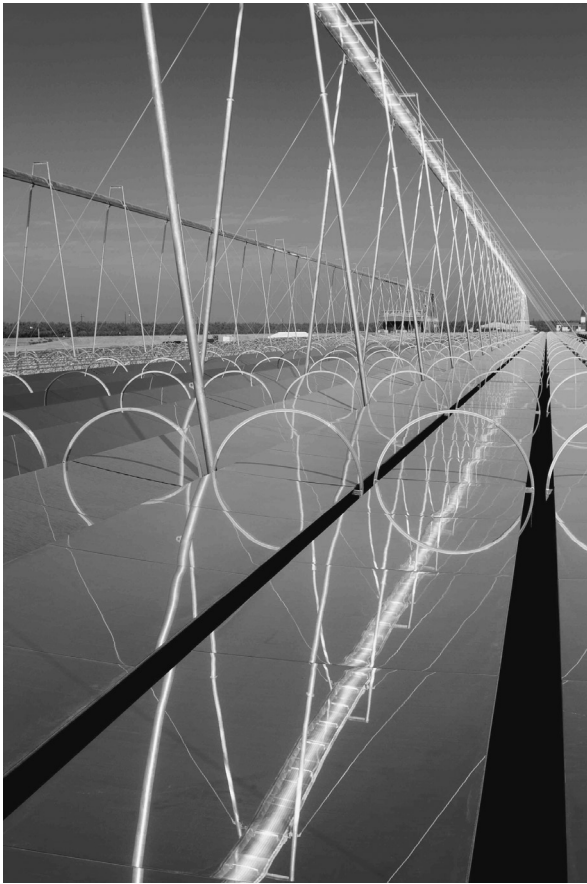
FIGURE 7.11 Close-up of mirrors (each 2 m wide) and receiver tube, which is 18 m above ground, Kimberlina plant. (From Sandia Labs.)
