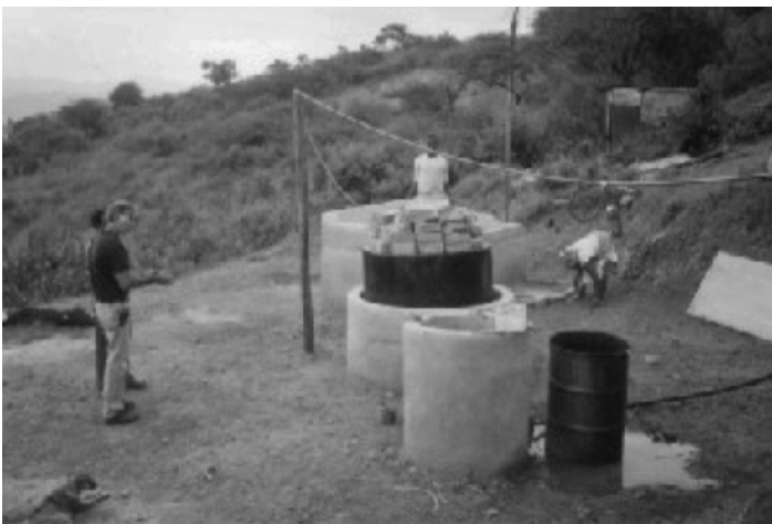
FIGURE 10.15 Floating roof biodigester in South Africa. (Courtesy of Solar Engineering, South Africa.)
