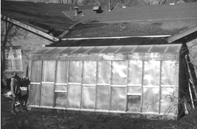
FIGURE 5.7 Attached greenhouse at Amarillo Children’s Home that was constructed by volunteers at AEI workshop.
