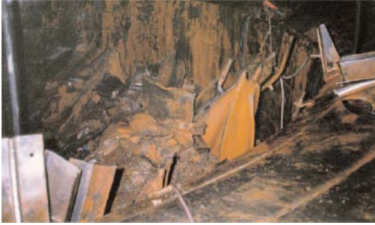
Figures 14 Internal damage
