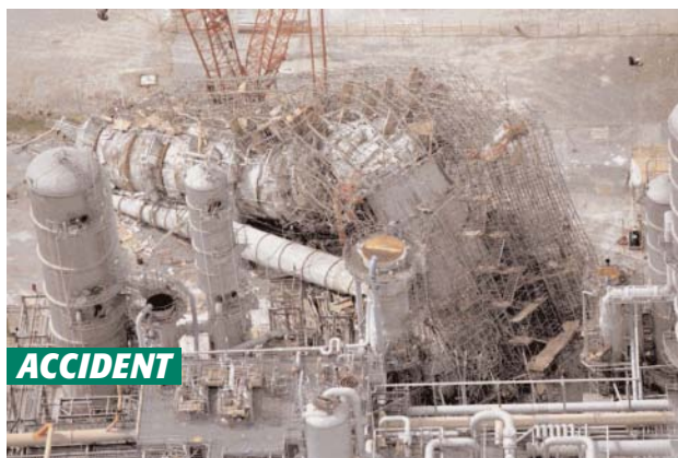
Figure 13 This column was completely destroyed by a pyrophoric fire. The fire happened during the replacement of the carbon steel structured packing, which involved cutting out the old column internals and removing each bed of packing. Despite persistent attempts to extinguish the fire, the incident progressed to the point where the splitter fell over early the next morning.
