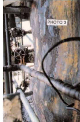
Bulge on shell
