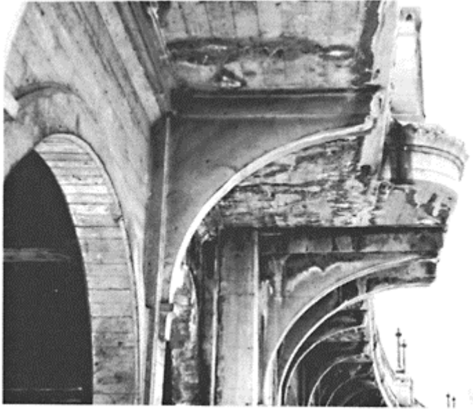
Fig. 2. Soffit of bridge deck shows evidence of extensive leakage
