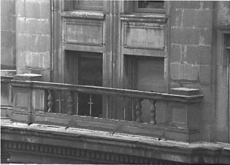
Fig. 2. Spalling of balusters was so severe that many were removed
