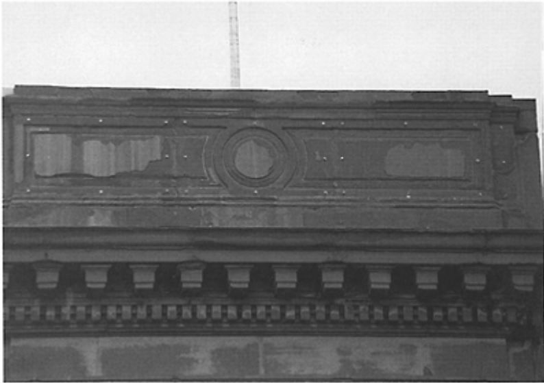
Fig. 1. Exfoliation of stone at building parapet
