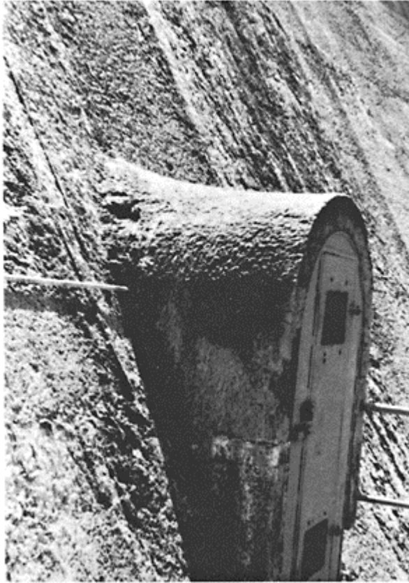
Fig. 9. Surface exfoliation and calcium deposits
