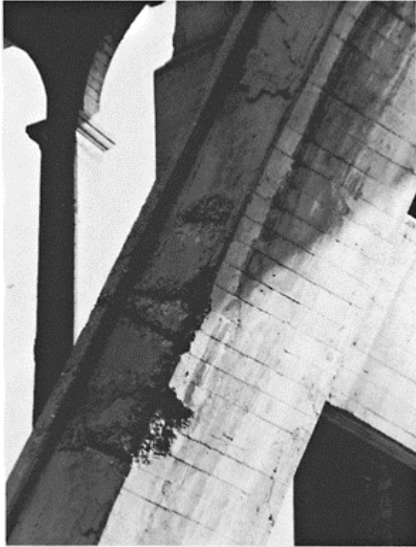
Fig. 3. Spalling and corrosion at arches. Large sections of reinforcing steel are exposed
