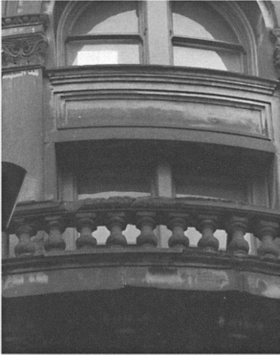
Fig. 6. Spalling of surface crust at balustrade railing and watertable edge
