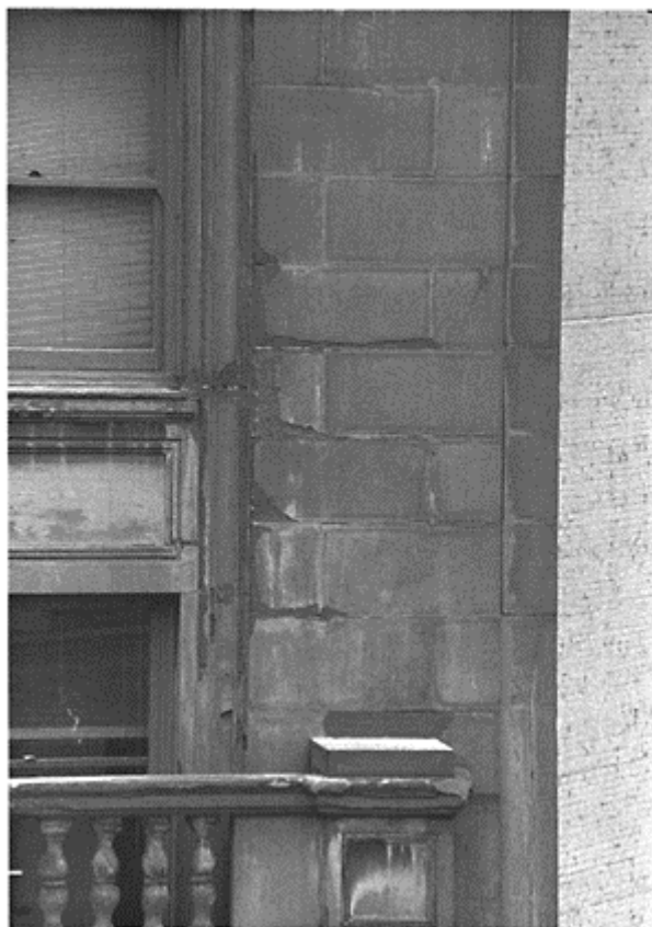
Fig. 5. Cracking and spalling at stone edges from expansion of surface crust
