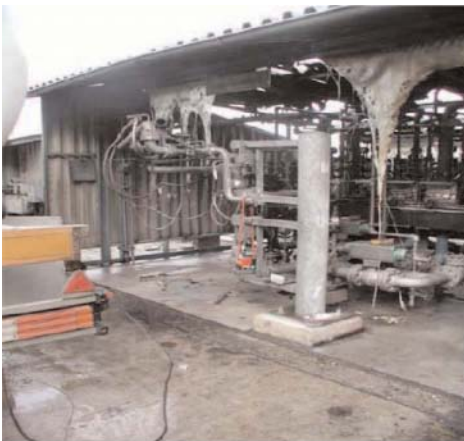
Figure 43a LPG loading station after fire.
