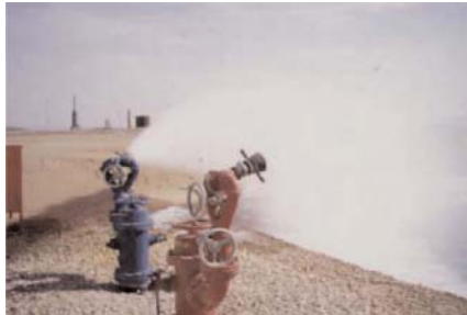
Figure 71 Monitors set to a wide angle spray to assist in the dilution of a gas release near the source.
