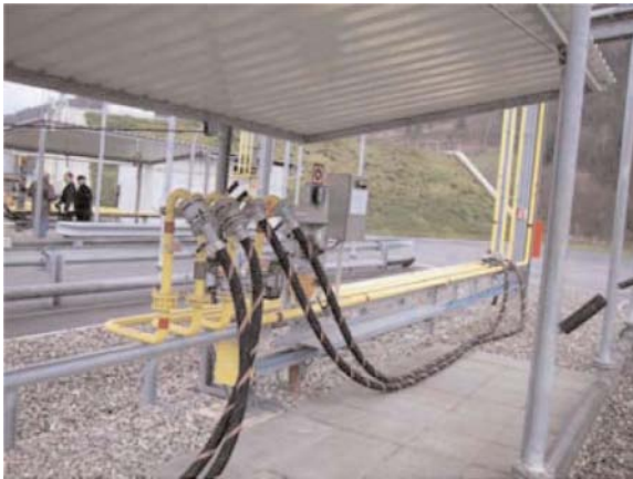
Figure 44 Example of road carloading station using flexible hoses.
