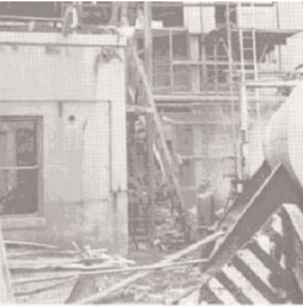
Figure 7 Fuel gas, leaking from a ruptured 3/4-inch line, accumulated in this pump room and ignited. The resulting explosion caused the damage shown. The line ruptured when water froze in it.
