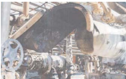
Figure 51b Ruptured heat exchanger.
