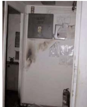
Figure 72b Electrical panel.
