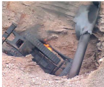
Figure 5b This bulldozer hit a gas pipeline. The driver was killed by the resultant fireball.
