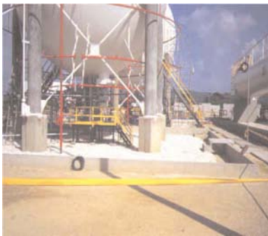
Figure 65 Example of lower fitted cooling spray rings for the lower hemisphere shell area to counter slippage and flame impingement effects.
