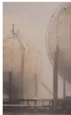
Figure 66 Example of a fixed ring cooling spray system. The nozzles may become blocked and they require regular testing and flushing to ensure total water coverage.
