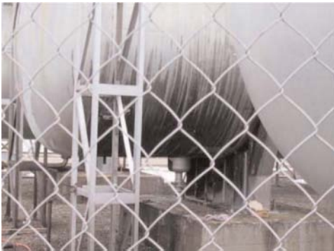
Figure 72a Draining point on the LPG vessel.
