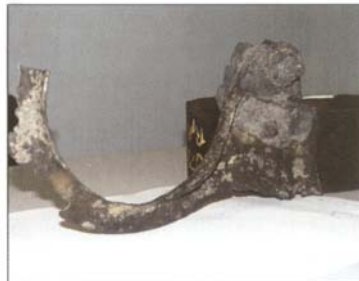
Corroded roof hanger.
