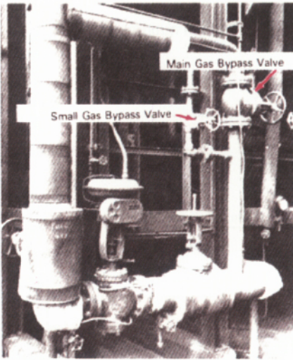
Figure 44b Gas bypass valves. The small gas valve is car-sealed (chain-locked) open during furnace operation to prevent flame-out.
