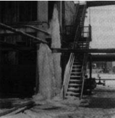
Figure 14 Freezing water leaks create hazardous working conditions.
