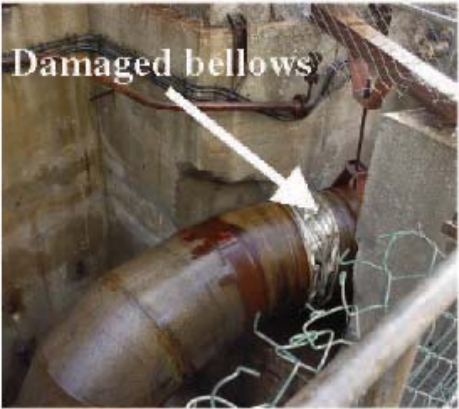
Figure 54 Flare drum lifted during a flood, damaging piping.
