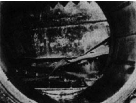
Figure 22 Damage caused in a combination tower when a small amount of water was flashed to steam.
