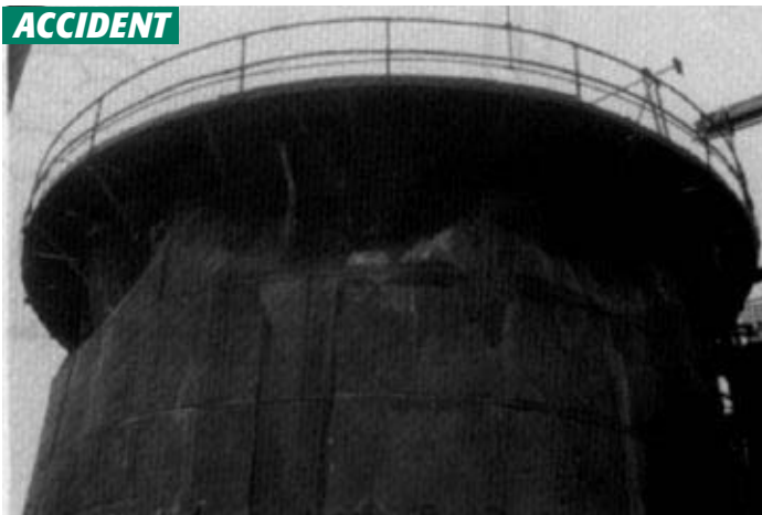
Figure 10 A vacuum vent and one open hatchway were not enough to prevent damage when steam condensed and pulled in the top two courses of this 35 ft (10 m) diameter by 21 ft (6 m) high wash tank.
