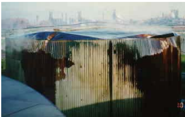
Figure 34b Atmospheric residue tank damaged by steam heating.
