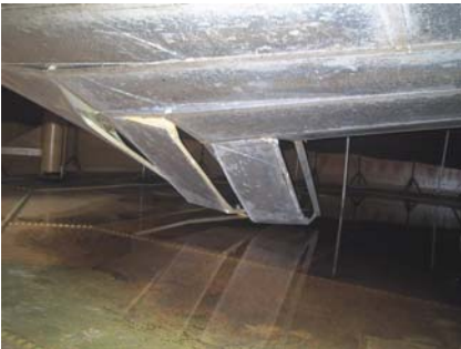
Figure 42b Collapse of a tank with internal floating roof due to excess weight applied.
