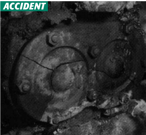
Figure 12 Pump cover plate was broken by freezing water.
