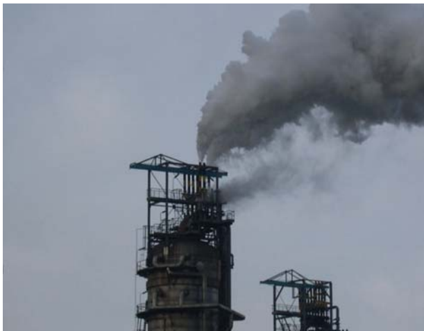
Atmospheric Relief Valves lifting on a CDU main tower
