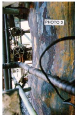
Bulge on shell
