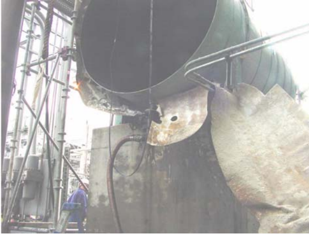
Figure 57b Ruptured vessel.
