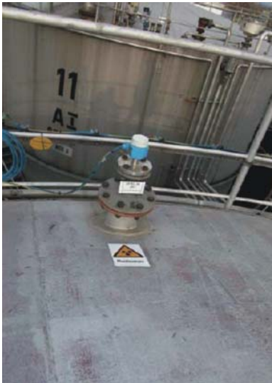
Level gauge on top of tank
