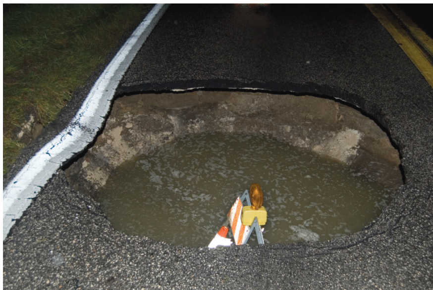
Plate 4 Harney Road sinkhole, Hillsborough County, Florida. This was caused by an underground rupture of a sewage pipe. Photo by Jason Polk
