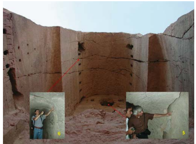
Fig. 25.46. Identification of monitored discontinuities in Giant Western Buddha niche
