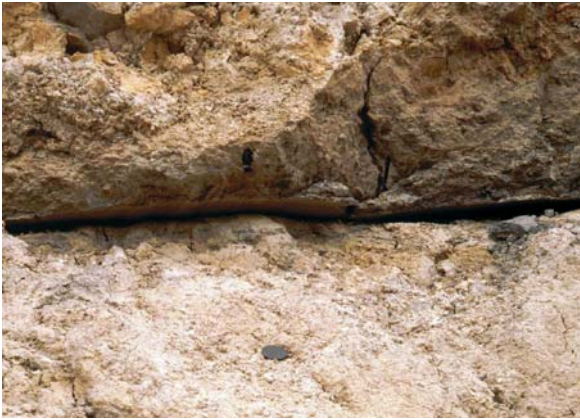
Fig. 2.15. Bedding-controlled slip surface in the Fairlight Clays (Sussex)
