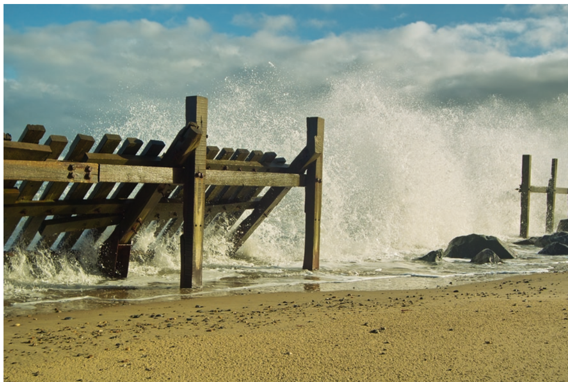
Fig. 3 Defences such as these are proving inadequate
