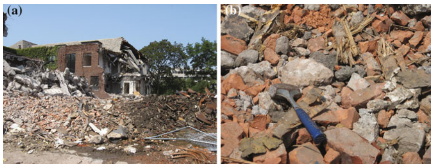
Fig. 2.2 Aging infrastructure is common in major urban areas worldwide: a building demolition during urban renewal; b demolition debris typical of that found in modern urban soils (wood, brick, mortar, concrete, cinder block, etc.). Photos by J. Howard
