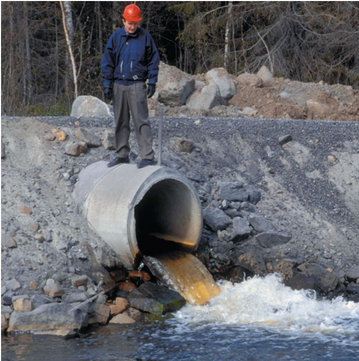
Figure 24.6 Urban stream erosion. Urbanization has adverse effects on streams due to excess and polluted runoff.
