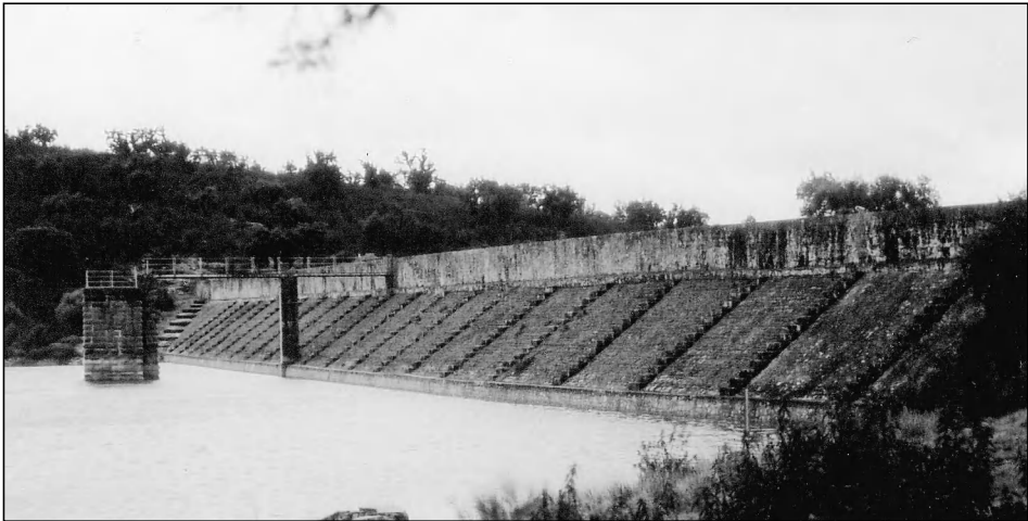
Figure 6.28 The dams of Prosperina (above) and Cornalvo (below), near Merida (Emerita Augusta). These are among the oldest dams still in use, seen from upstream (photos by CEHOPU (CEDEX), Miguel Otero).
