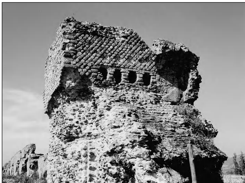
Figure 6.13 The head tank of the Garon siphon at Soucieu (Gier aqueduct); longitudinal and horizontal sections at the level of the openings, and seen from downstream, with the four openings that remain intact (photo by the author). This reservoir is raised 4 m above ground level. Its walls are 80 cm thick.
