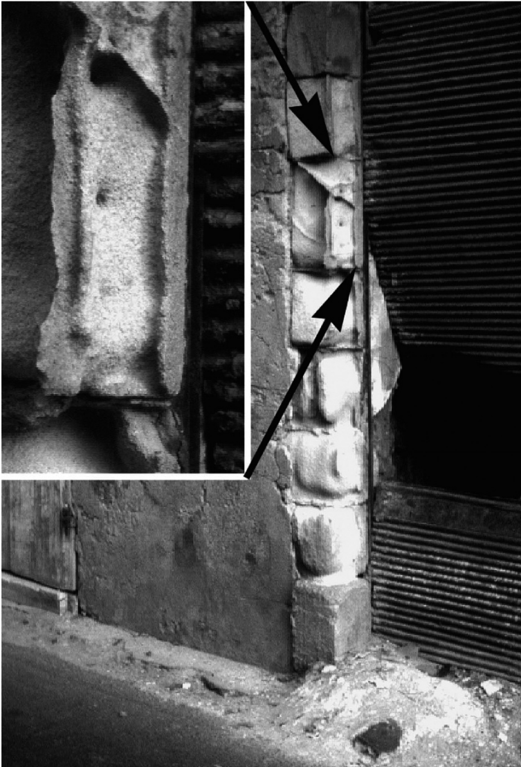
Fig. 11.10 Weathering of sandstone blocks
