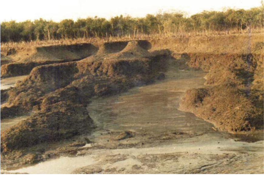
Fig. 3.4 Severe erosion near mouth of Thakuran at Dhanchi. The bank slopes down into gentle platforms. Note the conspicuous nature of erosional mud ridges
