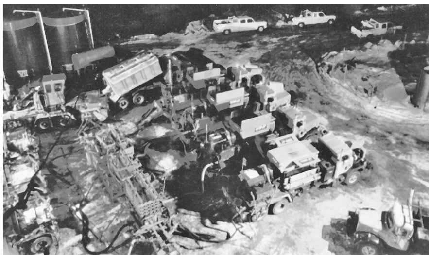
Fig. 6-19. Dowell equipment deployed around EE-2 for the MHF Test. Source: HDR Project photo archives
