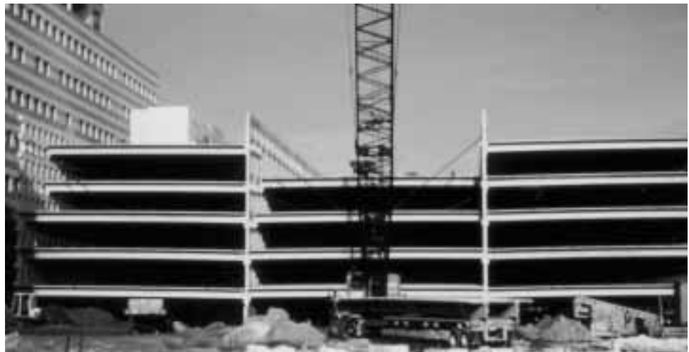
Figure 7-1 Crane in middle bay setting three bays at a time – bringing the building out in one sequence.
