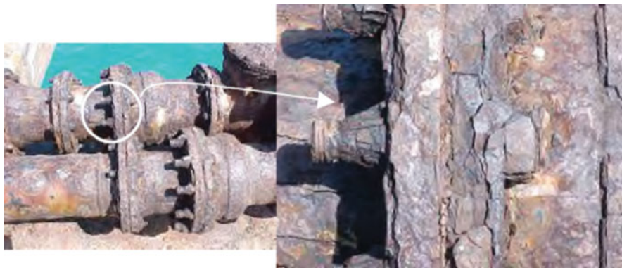
Fig. 1.3 Uniform corrosion (atmospheric attack) of a pipeline located on a concrete pier above the ocean water
