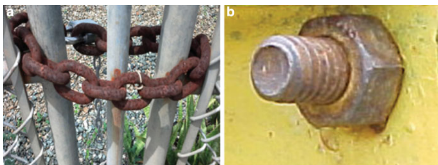
Fig. 1.4 Galvanic corrosion of a (a) steel alloy chain and (b) carbon steel bolt-nut coupling
