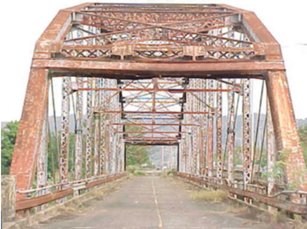
Fig. 1.2 Uniform corrosion (atmospheric attack) of a steel bridge
