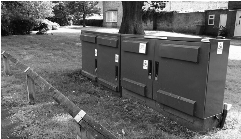
Figure 14.6 One of the energy storage management units installed on the streets of Bracknell as part of the Ofgem funded Thames Valley Vision smart grid trial. Image provided by Timur Yunusov.
