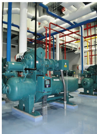
Industrial ammonia refrigeration system.
