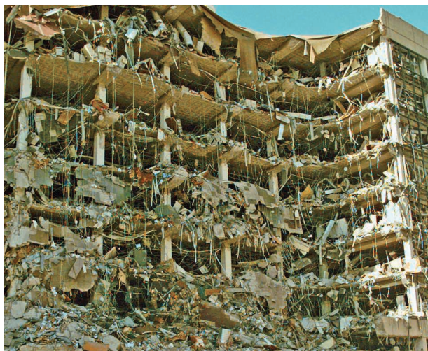
The Alfred P. Murrah building after a deadly explosion caused by an ammonium nitrate bomb.
