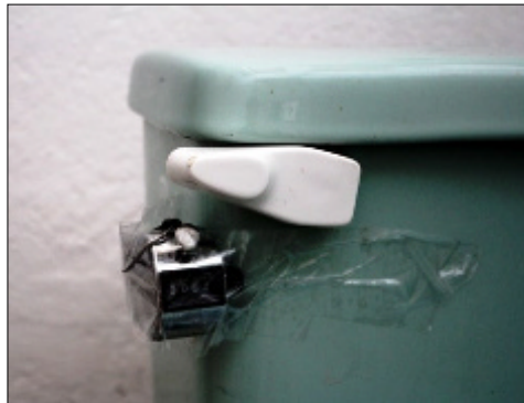
Figure 5.3-Picture of hand counter installed on toilets
