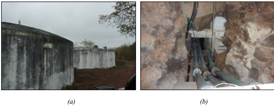
Figure 3.3-Pictures of (a) Storage tanks and (b) three pumps installed for extraction of brackish water at "La Camiseta".
