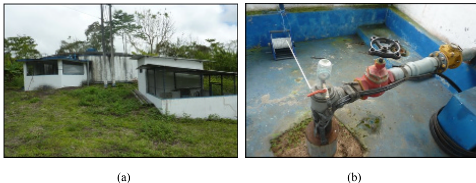
Figure 3.5- (a) Storage tank and pumping station and (b) extraction pump at Bellavista
