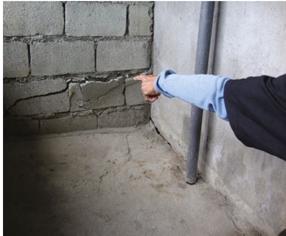
Fig. 6.4 A homeowner points to the cracked wall of his housing unit because of the gradual sinking of the ground. Source Author
