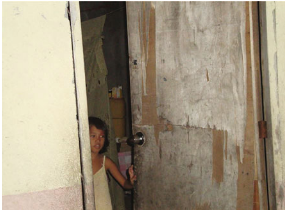
Fig. 7.3 Aling Bettyline’s sickly child opening the main door of the house. This house was just bought two years old, and yet one can see the deterioration and cracks due to the poor quality of the building materials and construction defects. Source Author
