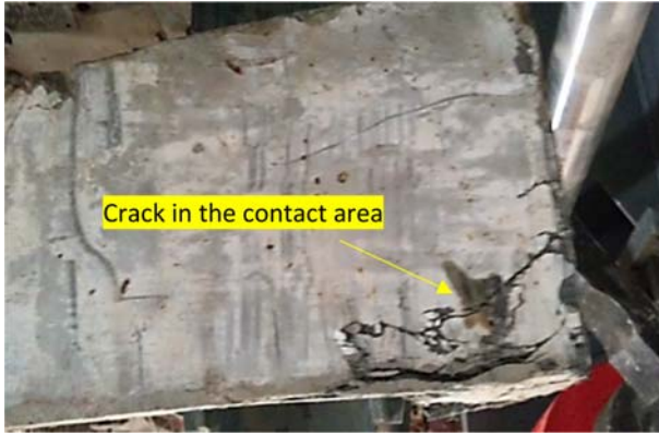
Figure 4.19 Boundary cracks on U2A.
