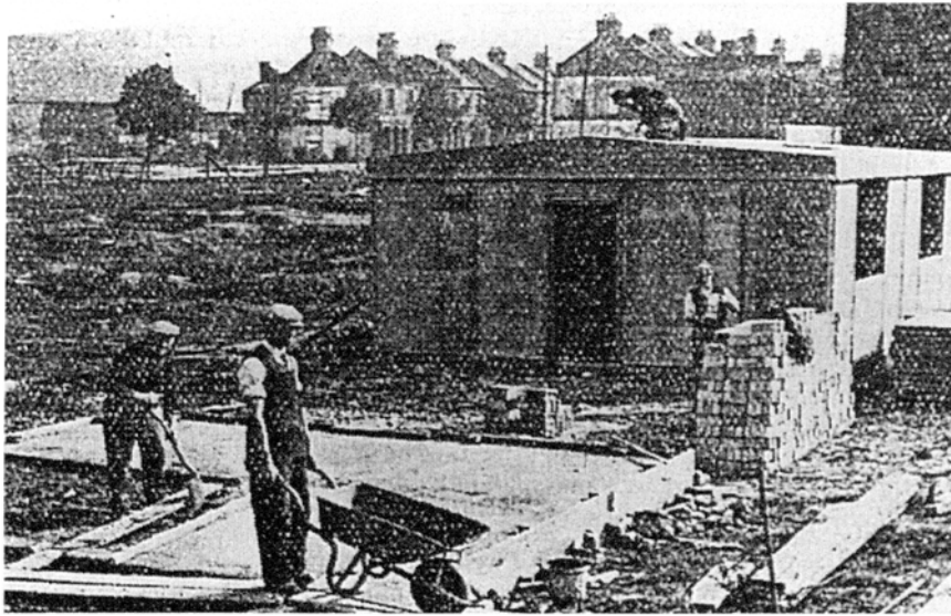
Figure 6.1. The Uni-Seco emergency hut, built in response to the damage caused by the V2 rocket bombs, under construction. (Source: The Builder , 22 September, 1944)
