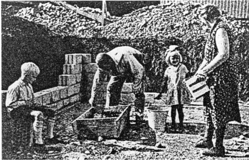
Figure 7.1. Swedish family at work on the foundations for a factory-made timber house. (Source: Architects' Journal , 31 May, 1945)
