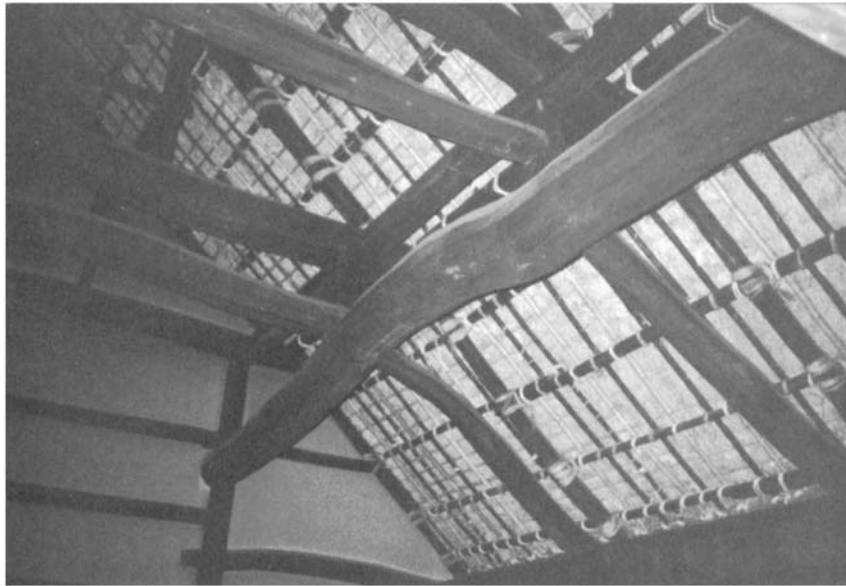
Figure 7.4 Natural wood beams and columns. Such natural materials have very good structural properties. Housebuilding techniques were similar throughout Japan.
