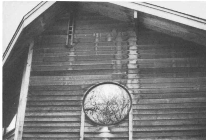
Figure 4.6 Sidewall moisture and external discoloration are evident on this cathedral ceiling house that has an inadequate air barrier.
