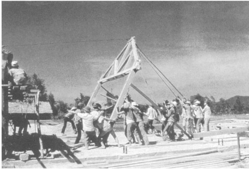
Figure 8.4 Builder training programme in Vietnam: participants raise the main roof frames for the first demonstration building, a primary school (from John Norton).
