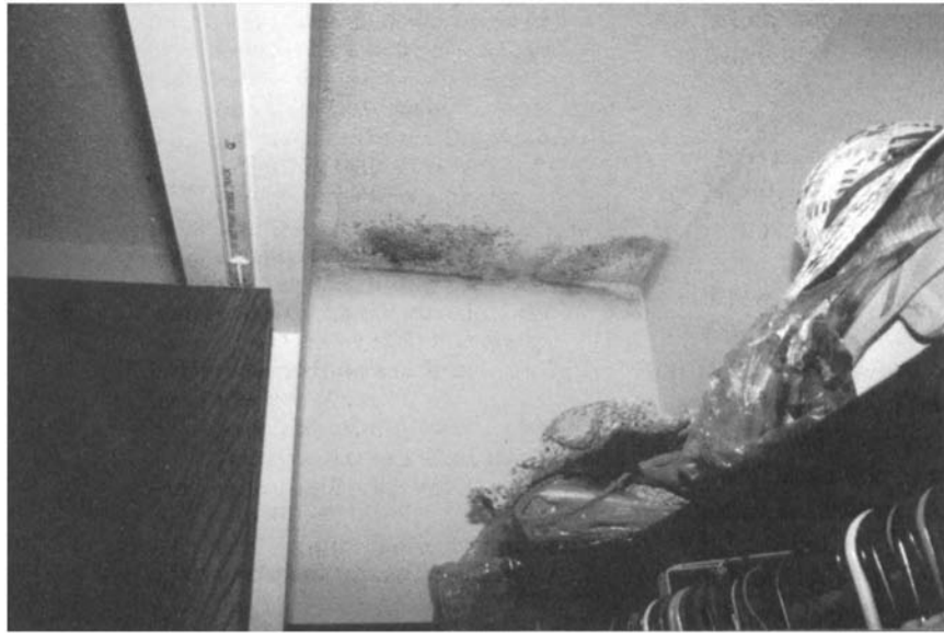
Figure 4.3 Mould and mildew are common occurrences where air circulation is poor and dew points are easily reached.
