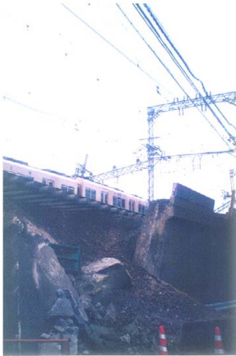
Fig. 12.13 Overturning of retaining wall during 1995 Kobe earthquake (near Hanshin Ishiyagawa Station)
