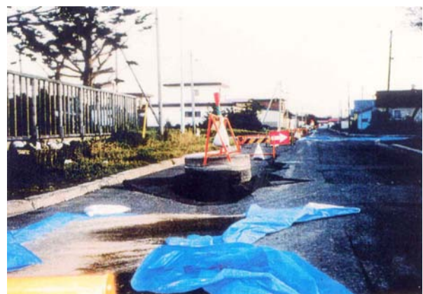
Fig. 17.18 Floating of manhole in Shibetsu
