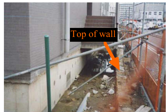
Fig. 24.83 Building foundation which was protected by underground walls from effects of lateral soil flow (Shimagami Pumping Station, Kobe; Photograph by Prof. Koseki)
