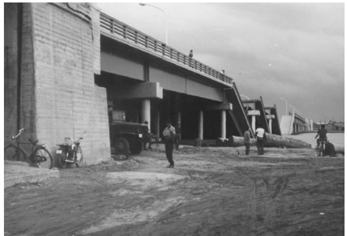
Fig. 24.64 Fallen Showa Bridge crossing Shinano River (Department of Civil Engineering, University of Tokyo)
