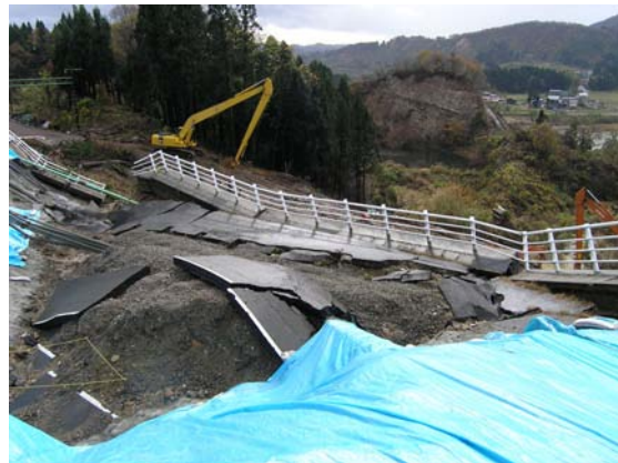
Fig. 14.24 Significant subsidence of road embankment resting on small valley topography caused by 2004 Niigata-Chuetsu earthquake
