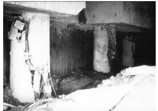
Fig. 24.7 Damage of piles caused by lateral soil flow (by Prof. K. Tokimatsu)
