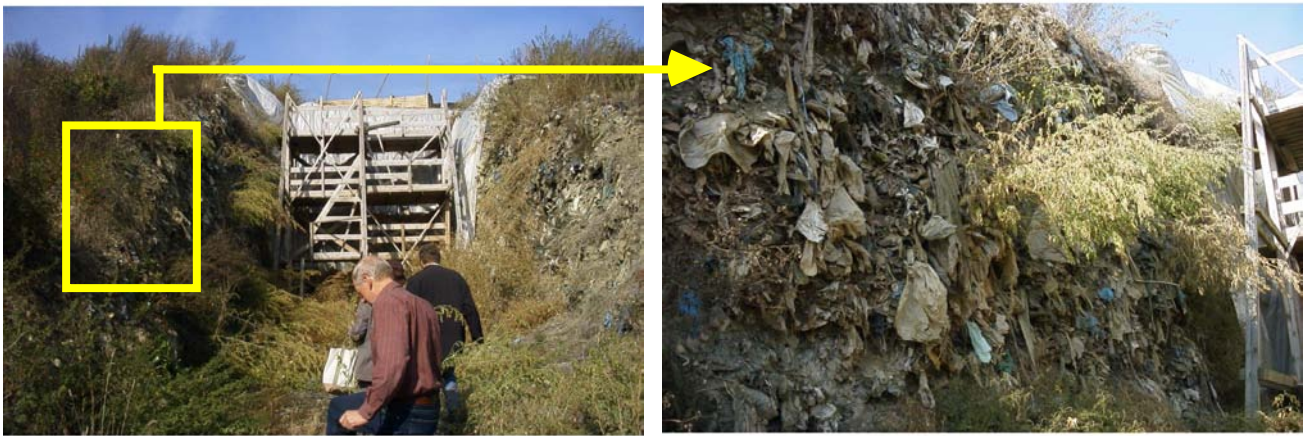
Fig. 10.75 Vertical and stable cliff in landfill near Göttingen, Germany
