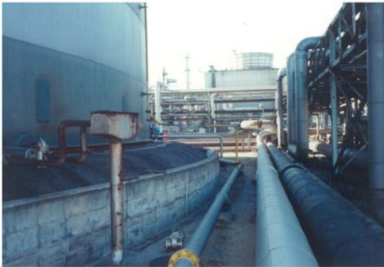
Fig. 26.24 Narrow space in oil refinery plant
