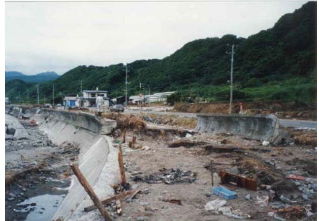
Fig. 16.59 Sea wall destroyed by retreating tsunami water (1993 Hokkaido Nansei-oki earthquake)
