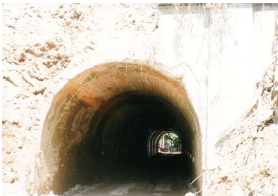
Fig. 16.36 Compressed arch of tunnel in Taiwan (1999)
