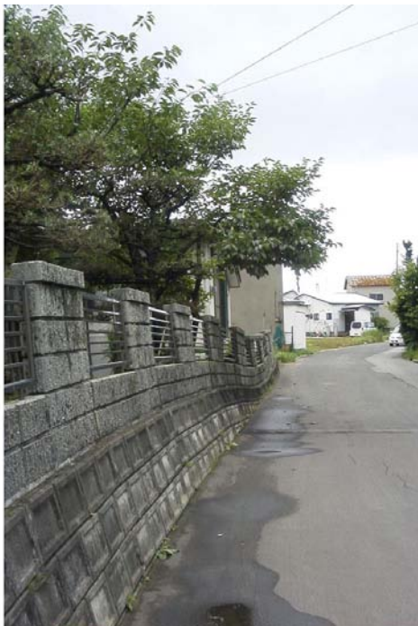
Fig. 17.60 Distortion of retaining wall due to subsurface liquefaction (Noshiro City in Akita, Japan)
