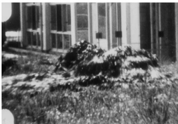
Fig. 25.59 Subsidence of Niigata Airport terminal building into liquefied subsoil (from motion picture by Mr. F. Yuminamochi)
