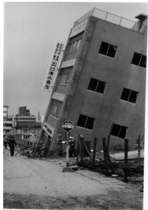
Fig. 17.2 Subsidence and tilting of building in Niigata (Department of Civil Engineering, University of Tokyo)
