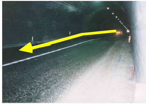
Fig. 16.32 Wave-like distortion of tunnel pavement during the 1990 Manjil earthquake in Iran
