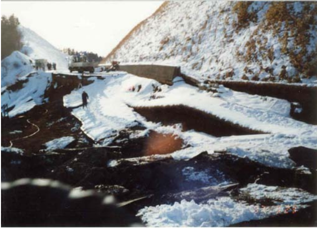
Fig. 14.43 Failed shape of Itoizawa road embankment in 1993
