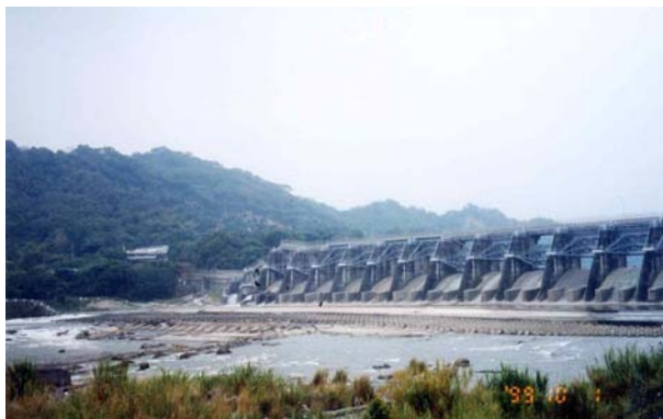
Fig. 16.9 Destroyed Shih-kang Dam
