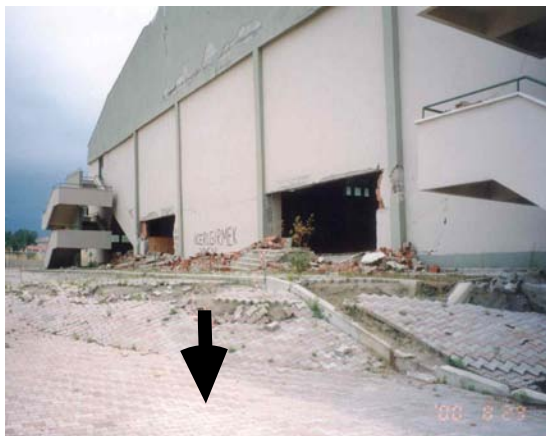
Fig. 16.47 Fault action at surface of Gölcük
