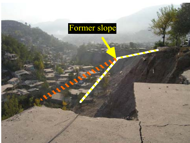
Fig. 15.5 Collapse of dry slope in Muzaffarabad, Pakistan
