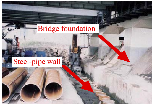
Fig. 26.17 Installation of steel-pipe wall for protection of bridge foundation from lateral soil movement (Photo by Prof. S. Yasuda)
