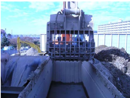
Fig. 26.139 Production factory for mixing waste soil with cement, gravel, and water
