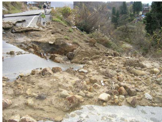
Fig. 14.9 Failure of road embankment during the 2004 Niigata-Chuetsu earthquake
