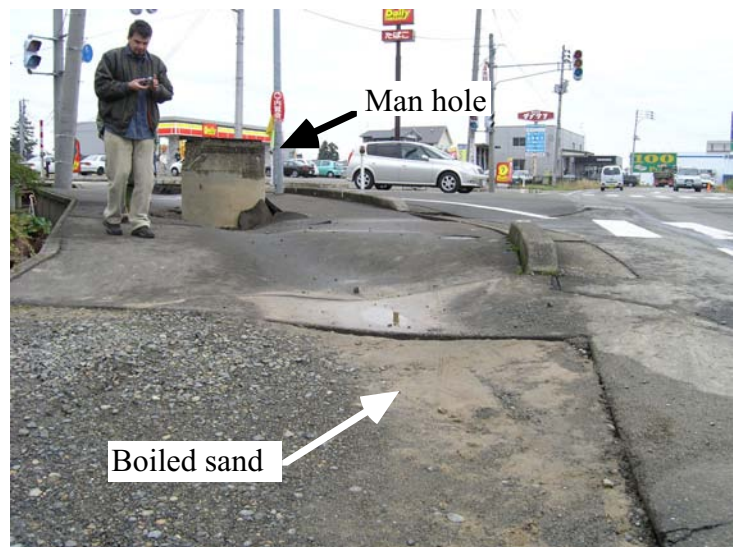
Fig. 26.137 Uplift of sewage manhole and boiled sand as evidence of backfill liquefaction (Ojiya City, 2004 Niigata Chuetsu earthquake)
