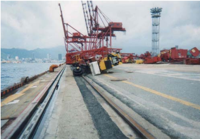
Fig. 24.33 Distortion of caisson quay wall in Kobe
