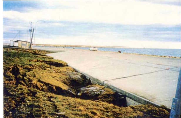
Fig. 17.21 Liquefaction damage at Hanasaki
