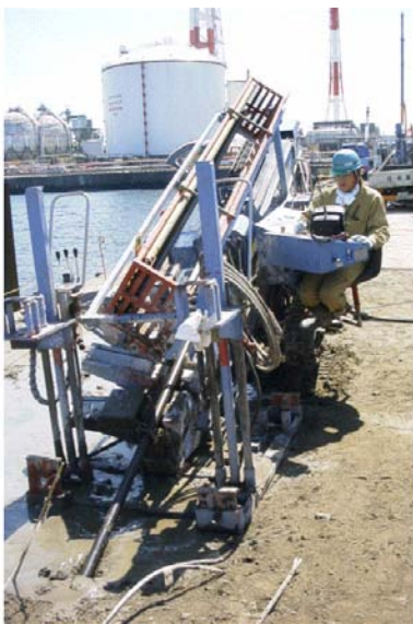
Fig. 26.119 Inclined drilling of bore hole for grouting under existing structure (Toa Corporation)
