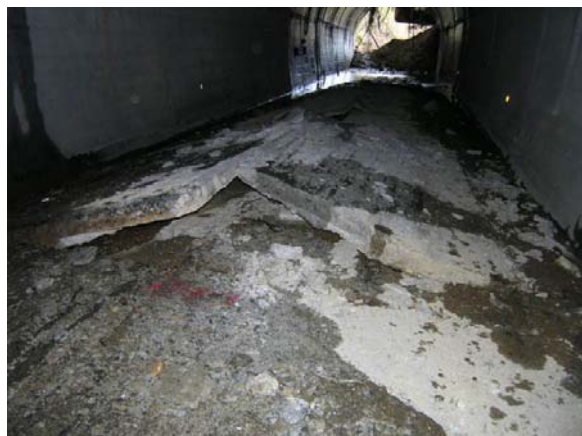
Fig. 13.24 Distorted shape and buckling of pavement in Haguro Tunnel, Niigata-Chuetsu
