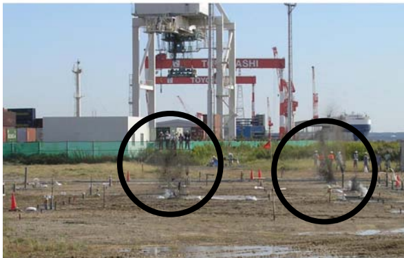
Fig. 26.141 Blasting and leaking gas from bore hole
