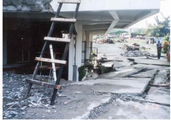
Fig. 17.3 Subsidence of building in Dagupan City
