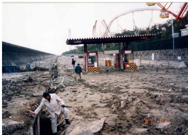
Fig. 20.9 Liquefaction of gravelly ground
