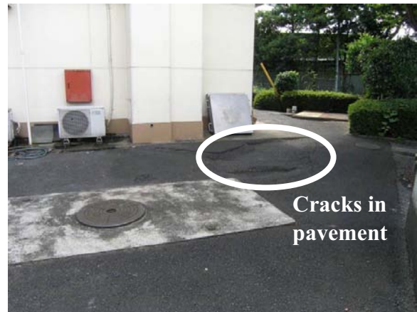
Fig. 9.41 Differential settlement around building
