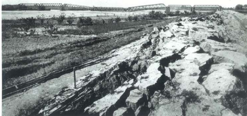
Fig. 14.14 Cracks at the top of Nagara River dike caused by 1891 Nobi earthquake (Photo supplied by Ministry of Construction)
