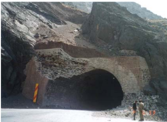
Fig. 16.34 Damage at entrance of tunnel (Manjil earthquake)
