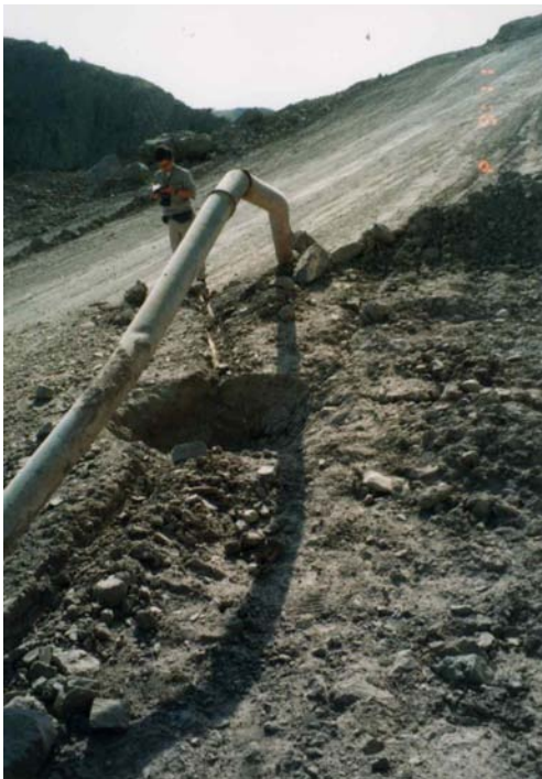
Fig. 16.38 Buckling of pipeline due to fault action (Manjil earthquake, Iran, 1990)
