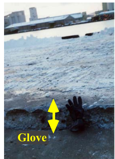
Fig. 26.89 Subsidence of ground with gravel drains relative to stable quay wall (Kushiro Harbor, 1993)
