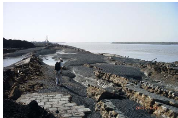
Fig. 17.12 Shear failure of harbor fill in Navrakhi harbor of India
