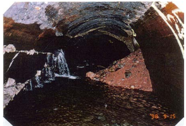
Fig. 16.37 Water tunnel distorted by crossing fault (by N. Yoshida)
