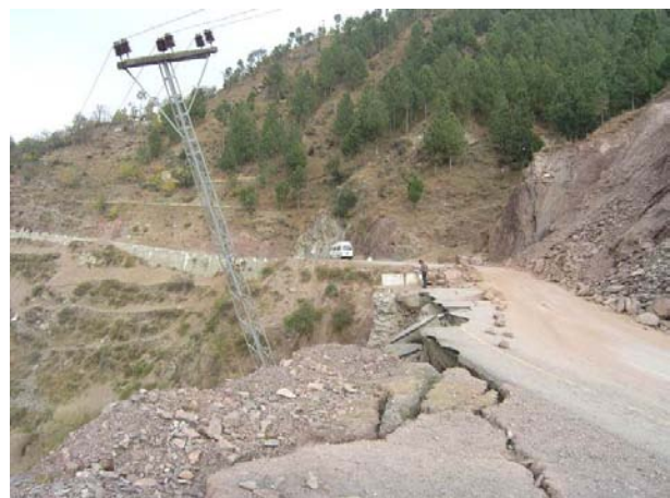
Fig. 15.8 Collapse of slope surface and road shoulder near Barakot of Pakistan
