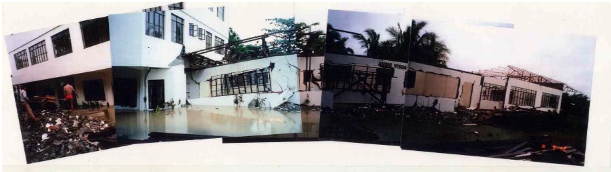
Fig. 17.4 Reduced subsidence of lighter annex
