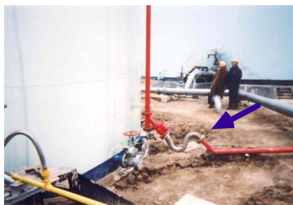
Fig. 17.33 Flexible joint of oil storage tank that absorbed heavily subsidence of tank
