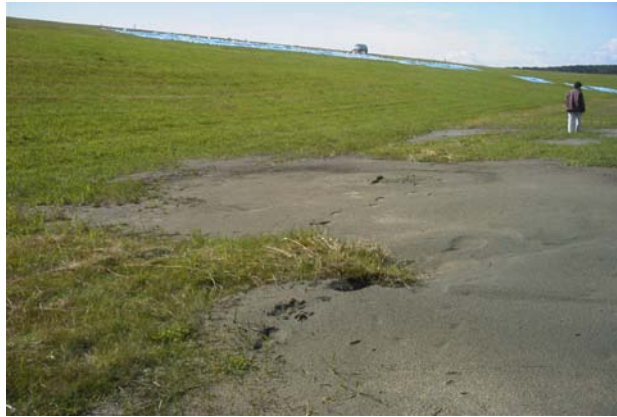
Fig. 17.13 Minor liquefaction near Tokachi River dike in 2003
