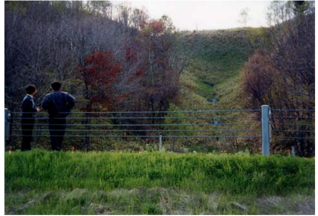
Fig. 14.44 Small creek at the place of embankment failure (Photo taken by T. Honda in May, 2000)
