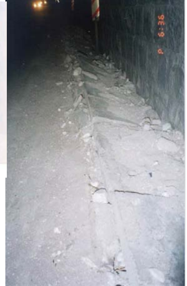
Fig. 16.33 Distortion of cover stone of drainage trench due to reduced width (Manjil earthquake)
