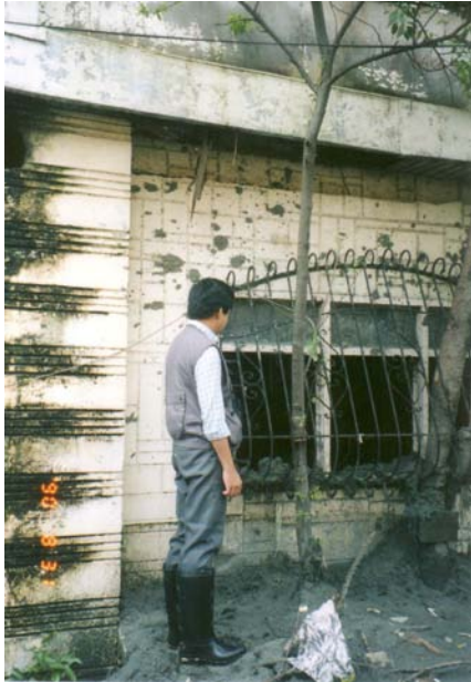
Fig. 18.4 Ejected sand on wall (Dagupan, 1990)
