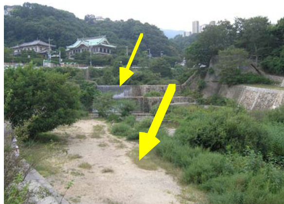
Fig. 26.5 Dams of debris in river channel
