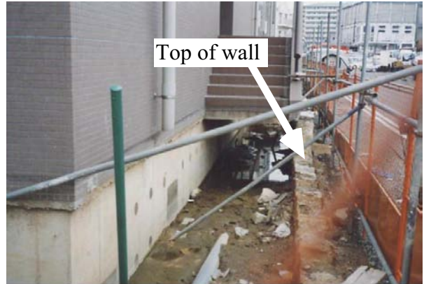
Fig. 26.11 Shimagami pumping station behind quay wall in Kobe (photograph by Prof. J. Koseki)
