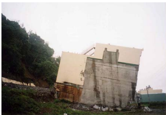
Fig. 16.11 Building resting immediately on fault (水源路 ChiChi earthquake in Taiwan, 1999)
