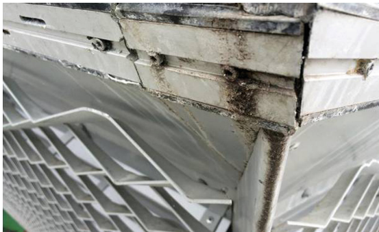
Fig. 8. Corrosion on the facades of Dokk1.
