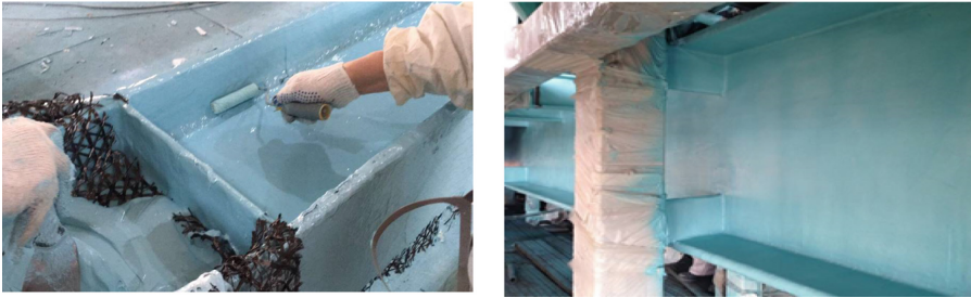
Fig. 2. Application of fire-retardant coating Firetex® M93/02 (left) and Firetex M90, Sherwin-Williams® 11 mm. Modules for YAMAL LNG. Photos were provided by Muehlhan Morflot LLC and LLC Osoran.
