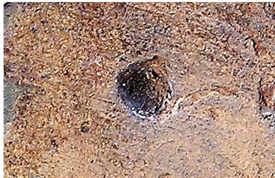
Fig. 2. Ulcerative individual corrosion defect of the first zone in the vertical steel tank.
