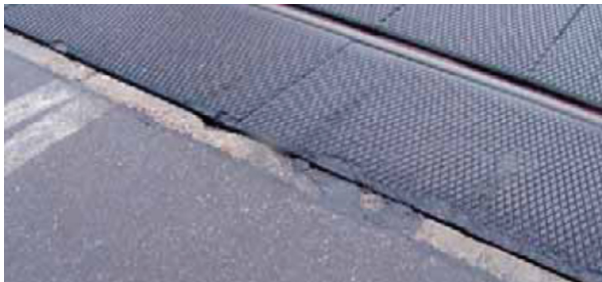
Fig. 6. Example of road pavement damage due to the inadequate radius of vertical curve [9].
