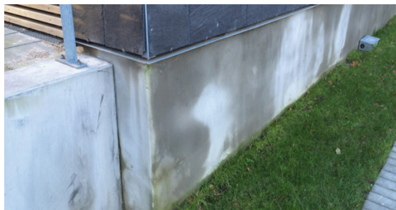
Fig. 1. The formation of traces of moisture on the surface.
