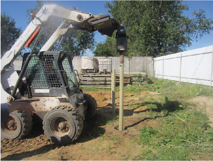
Fig. 4. Drilling of bored composite piles with a pultrusion fiberglass pipe (Source: Author’s research).
