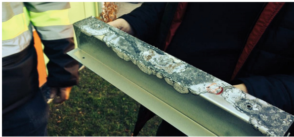
Fig. 4. Formation of the metal structure corrosion.
