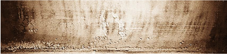
Fig. 3. Multiple ulcerative corrosion damage of the T-butt weld in the vertical steel tank.
