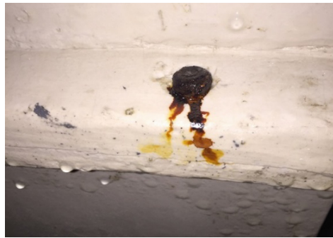
Fig. 5. Corrosion on fasteners elements.
