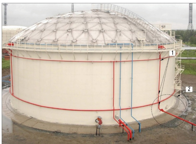
Fig. 1. Overall view of the fire-fighting pipeline and VST-20000 connecting assembly: 1 – pipeline connections with the VST wall, 2 – examined assembly.
