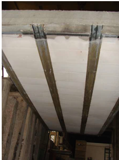
Fig. 6. Prototype No. 2 after the test, view of the lower (heated) side of the slab.
