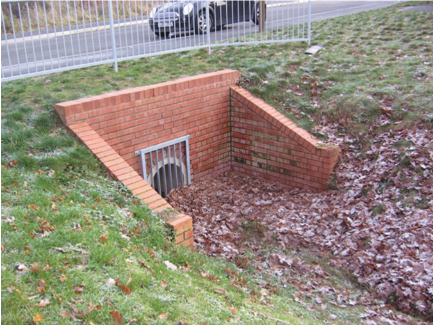
Figure 16.5 Storm sewer screen at the outflow of a SUDS management train, North Hamilton, Leicester (UK).
