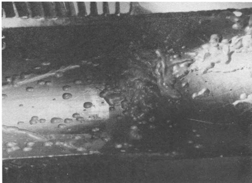
Figure 8.8: Corrosion at Tube Inlet Due to Missing Anodes
