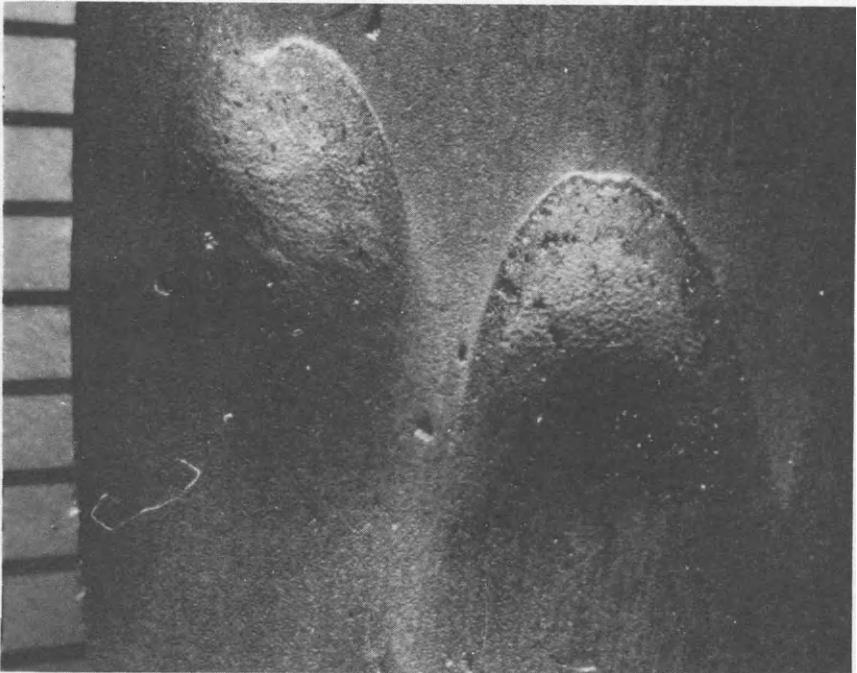
Figure 8.7: Erosion-Corrosion Attack at Tube Inlet Caused by Too High a Water Velocity
