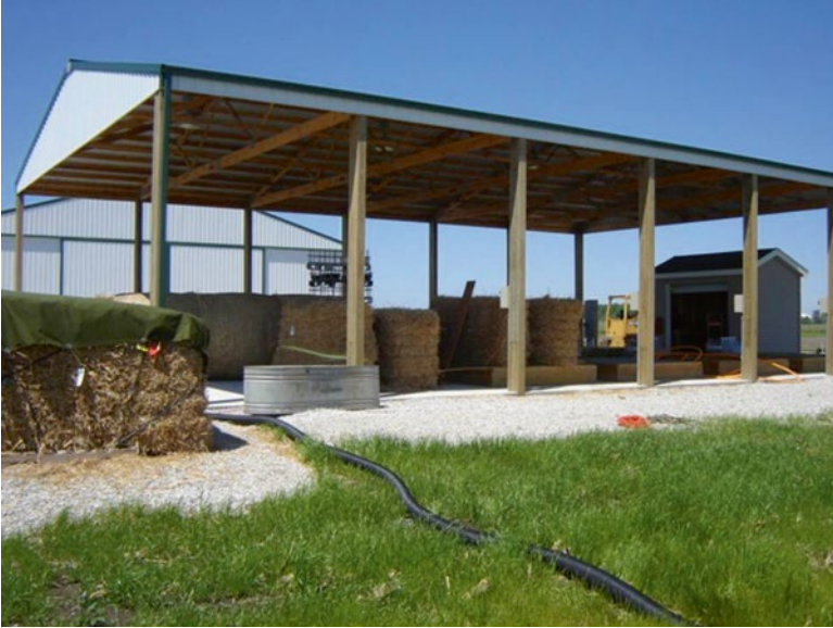
Fig. 7.4 On-farm covered storage of round bales in a shed without walls and any climate control mechanism
