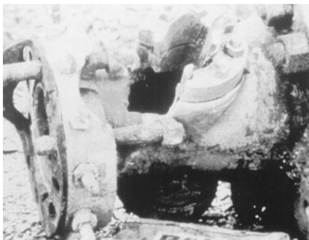
Fig. 5.3—Surface choke failure owing to erosion by formation sand (courtesy of Baker Oil Tools).
