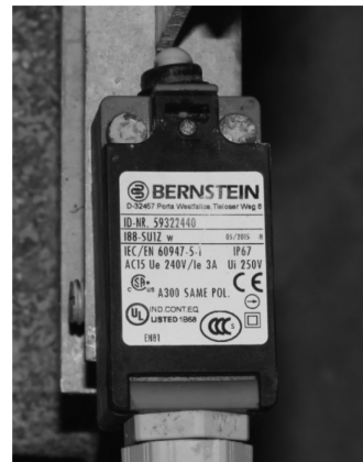
Figure 7. Electrical safety switch.
