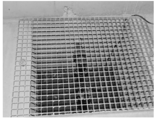
Figure 6. Sump with a pump for drawing water used to extinguish a fire.
