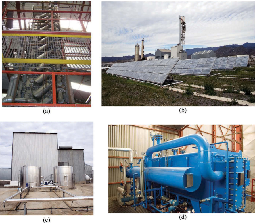
Figure 2.2. (a) Multi-effect distillation plant; (b) compound parabolic collector solar field; (c) thermal storage system; (d) double-effect LiBr-H 2 O absorption heat pump.
