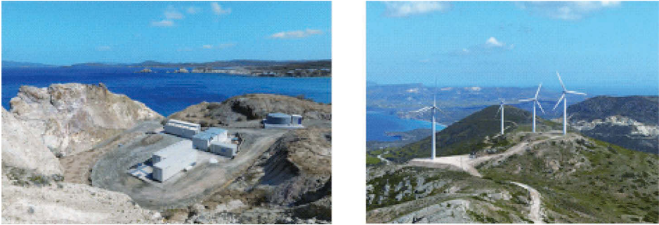
Figure 5.23. View of wind reverse osmosis plant on Milos island, Greece (Source: Bouzas and Relakis, 2010).
