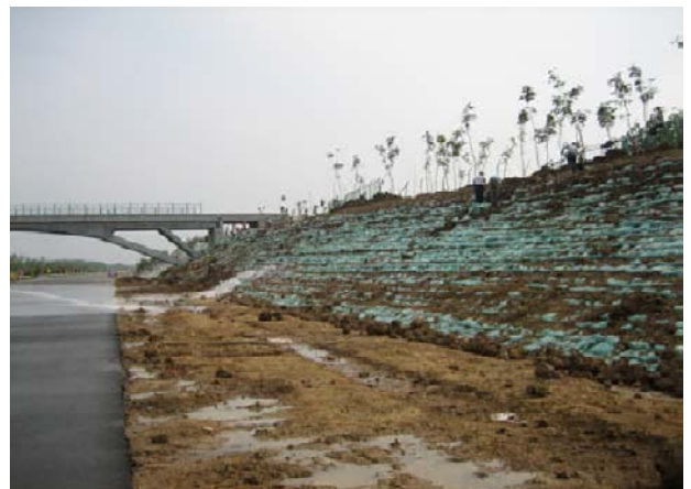
Fig. 12 Retaining walls of soilbags to protect expansive soil slope
