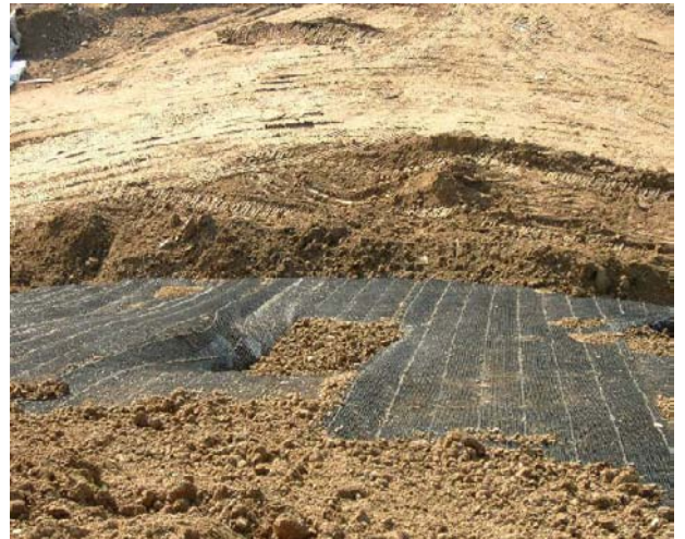
Fig. 8 Laying down of the topsoil layer. The hole previously excavated, where the tree will be planted, is clearly visible
