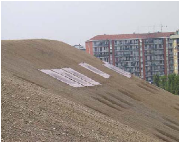
Fig. 5 Excavation of the holes for the trees, and specific protection of the holes with a nonwoven geotextile
