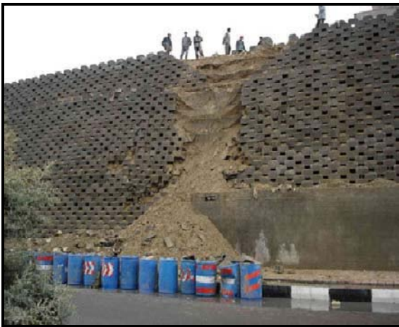
Fig. 3 Photo of collapse in the reinforced soil wall
