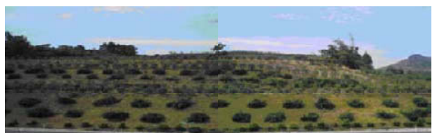
Photo 8 Effect photo of cut slope's landslide treated by three-step flexible support in a ramp of Ningming
