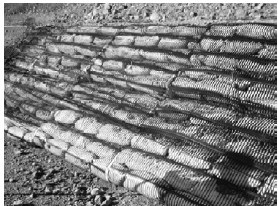
Fig. 4 View of the sacks wrapped around by the first layer of geogrids
