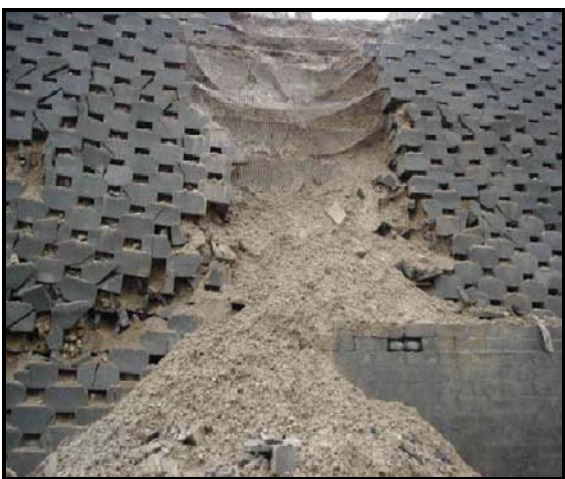
Fig. 4 Wall failure-geogrid layers visible
