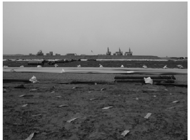
Fig. 5 Installation of liner system for the Laogang Municipal Solid Waste Landfill Project Phase 4
