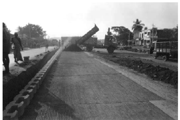
Fig. 10 View of geogrid reinforced segmental retaining wall under construction at km 292+412m VUP of NH5, Dharmavaram-Tuni Package
