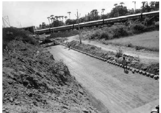
Fig. 9 View of geogrid reinforced segmental retaining wall under construction at Tuni ROB of NH5, Dharmavaram-Tuni Package
