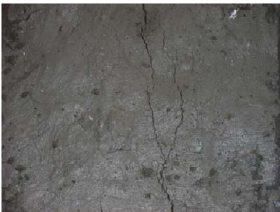
Fig. 11 Cracks on the embankment surface
