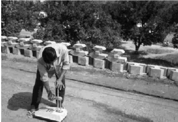
Fig. 16 In situ determination of soil density of compacted backfill for NH5, Dharmavaram-Tuni Package using Nuclear Moisture-Density Apparatus
