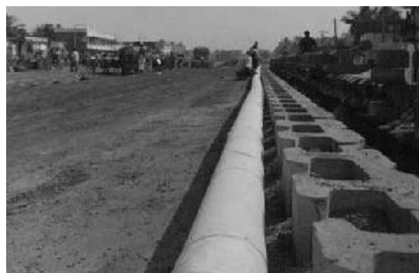
Fig. 4 Geotextile wrapped subsoil and aggregate drainage within and behind fascia units for NH5, Dharmavaram-Tuni Package
