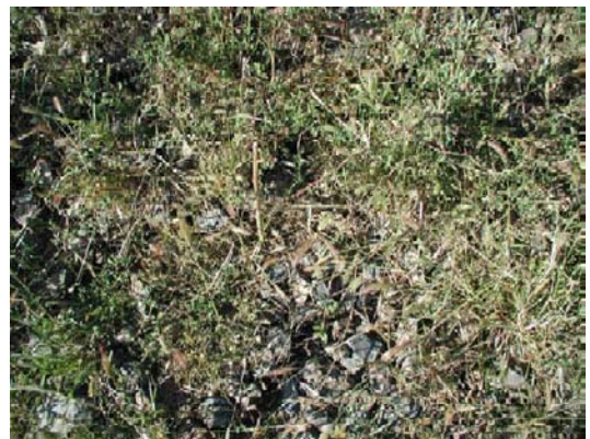
Fig. 4 The effect picture of geocell filled with gravel soil ecological slope protection
