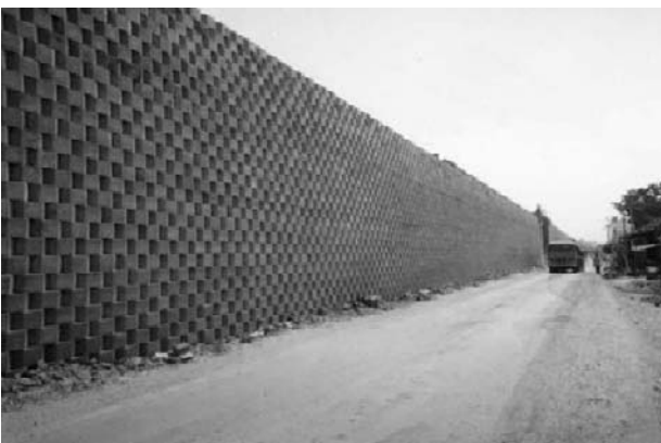
Fig. 13 Oblique frontal view of geogrid reinforced segmental retaining wall for NH5, Dharmavaram-Tuni Package
