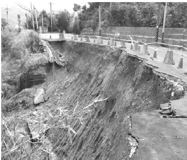
Fig. 5 RSS collapsed during an attack of typhoon
