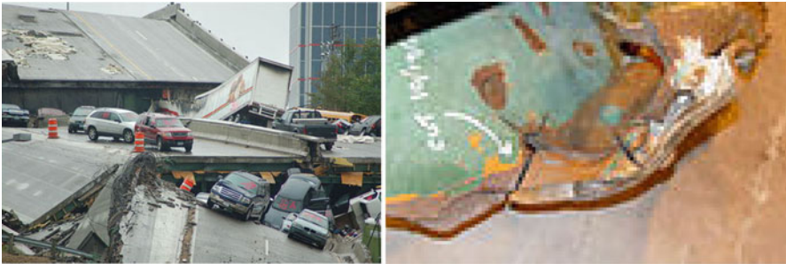
Fig. 6.13 Photo on left of the Minneapolis Bridge Collapse (courtesy US Coast Guard); Photo on right showing fracture in gusset plate (photo courtesy NTSB, 1990)
