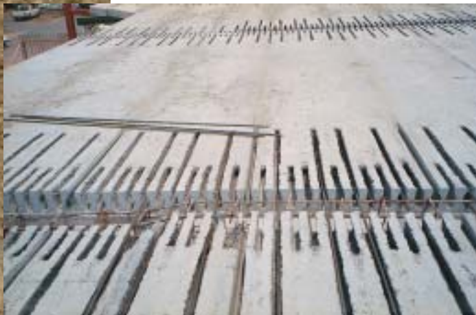
Figure 27 and 28: Tops of cores in hollow core slab opened up for reinforcement to form moment connection with beam.
