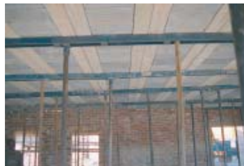
Figure 37: Propping under indicated positions.
